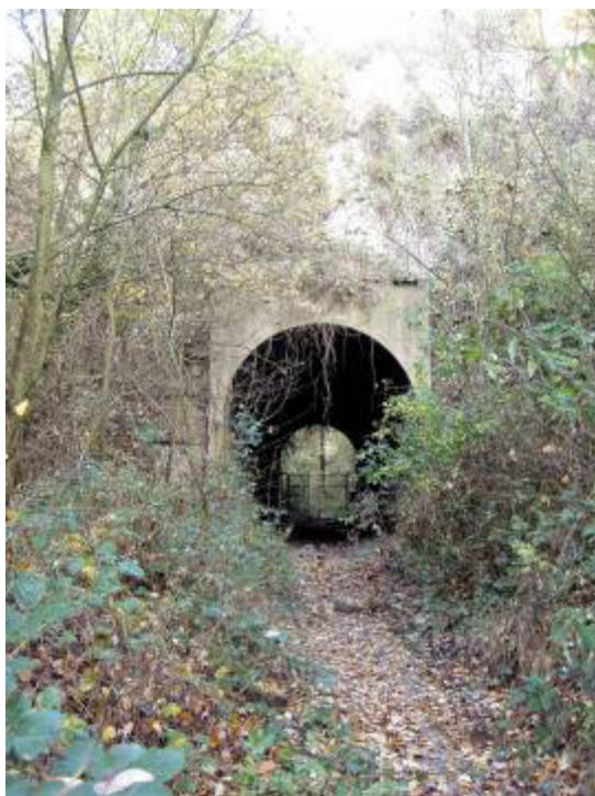
Fig. 28: Crayland Gorge Tunnel, Swanscombe Kent. This tunnel cuts through the chalk spine separating two quarries (photos:ECC/KCC 2004)
