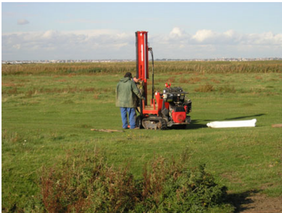
Fig. 9: Drilling at Binney Farm, Kent. The buildings on the horizon are on the Essex side of the estuary (Photo: ECC)
