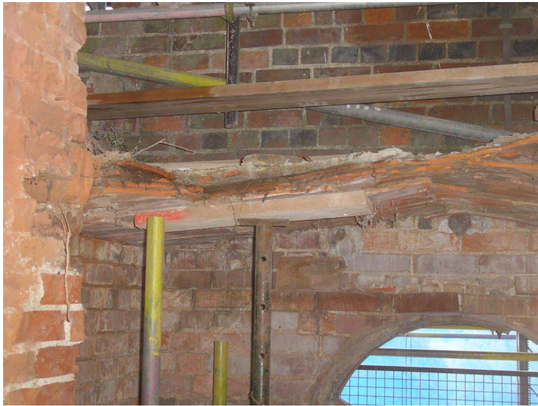
Plate 5. East side of roof showing tile construction topped by a concrete screed, looking southeast.
