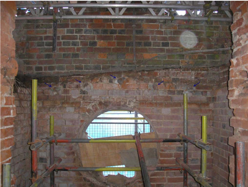
Plate 7. Roof removed leaving sloping scar on brick gable and small circular scars just below underside of roof indicated by arrows, looking south.
