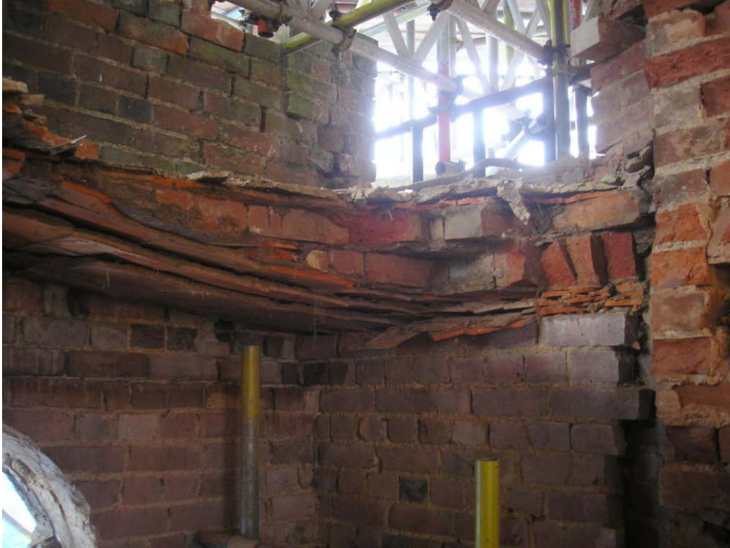
Plate 6. West side of roof showing brick and tile construction, topped by a concrete screed, looking southwest.
