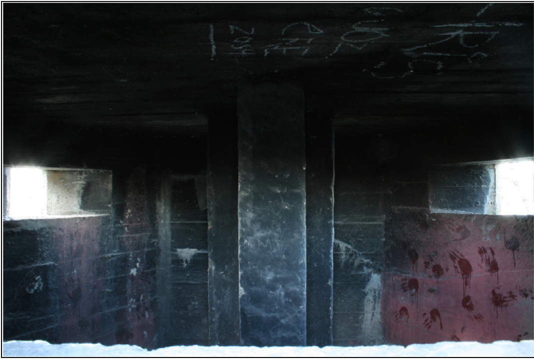
Plate 40 Internal view of pillbox, Building 11, showing ricochet wall and embrasures: OL-08007, looking west
