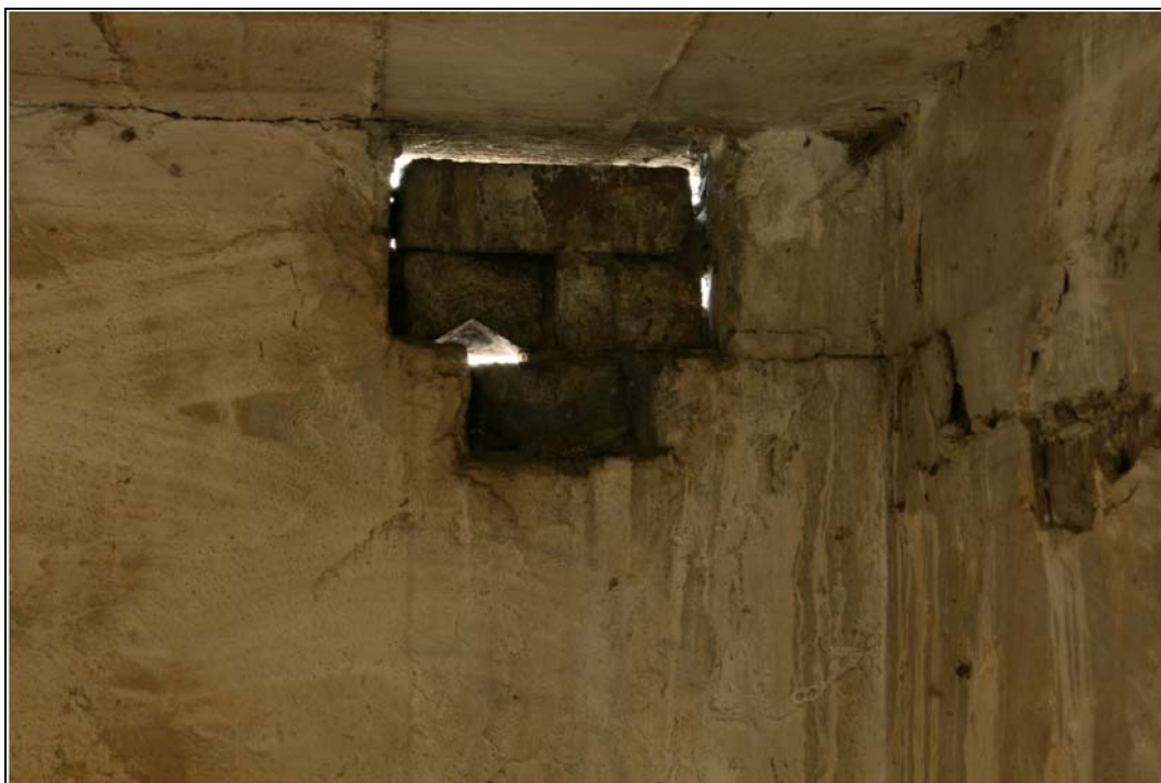
Plate 38 View of blocking detail in G2, radar station, Building 10: OL-01907, looking south-east
