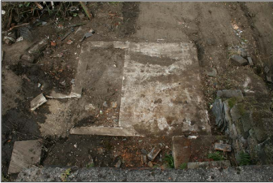
Plate 35 View of concrete base for generator, radar station, Building 10: OL-01907, looking north-west
