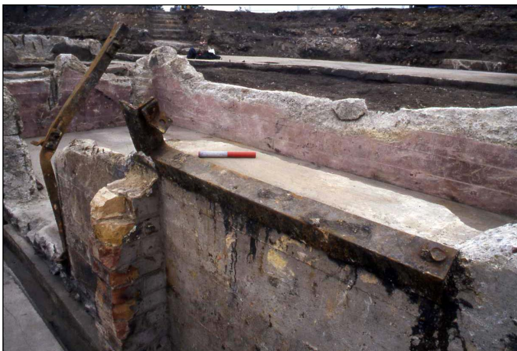
Plate 15 View of metal fixtures on window and door of cordite store, Building 3: OL-01907, looking south-west
