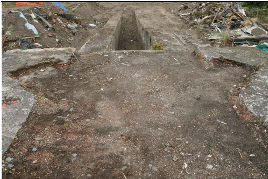
Plate 36 View of socket and ramps on radar station roof, Building 10: OL-01907, looking east
