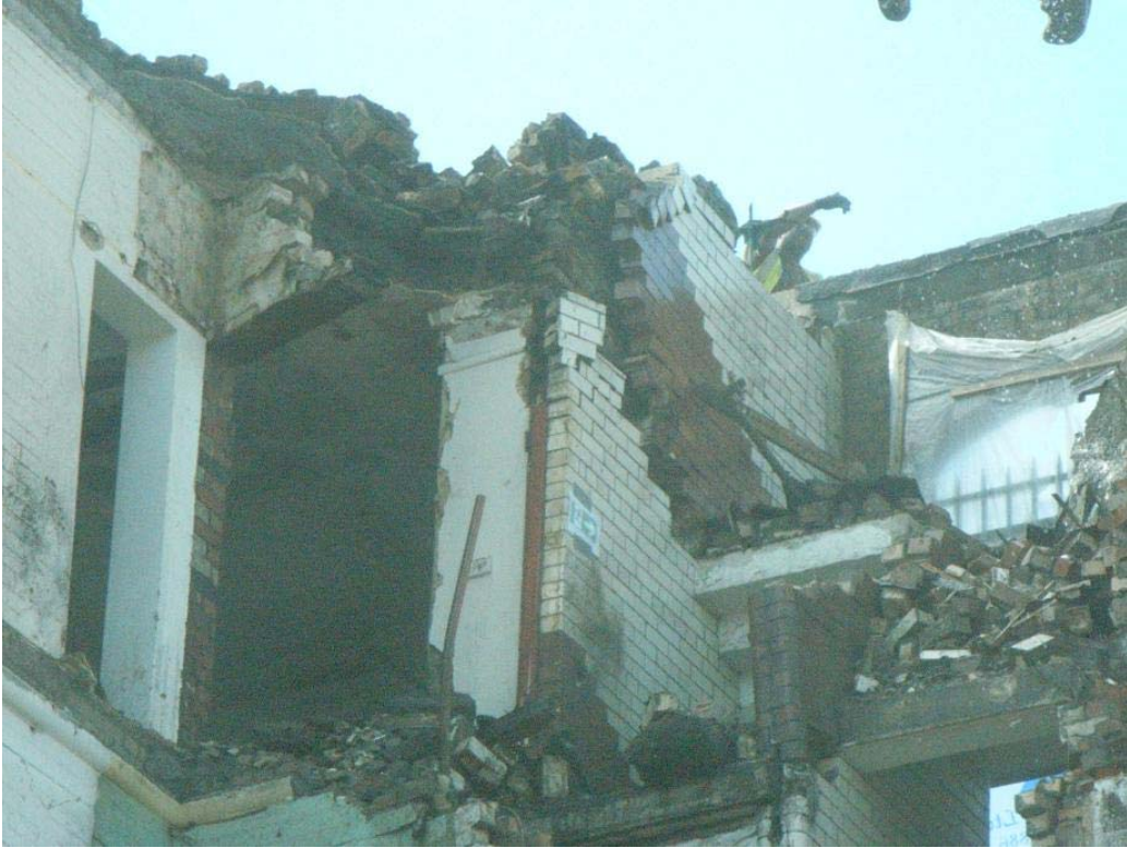
Plate 25: Recesses for stone steps in stairway wall of the Culross Building exposed during demolition
