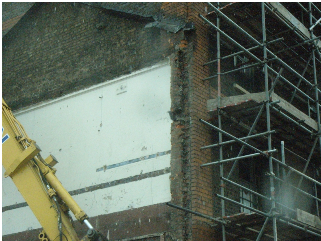
Plate 44: Ragged brickwork from bonded joint between Culross Hall (was left) and Culross Building (right) on the front (north-west) side of the buildings during demolition
