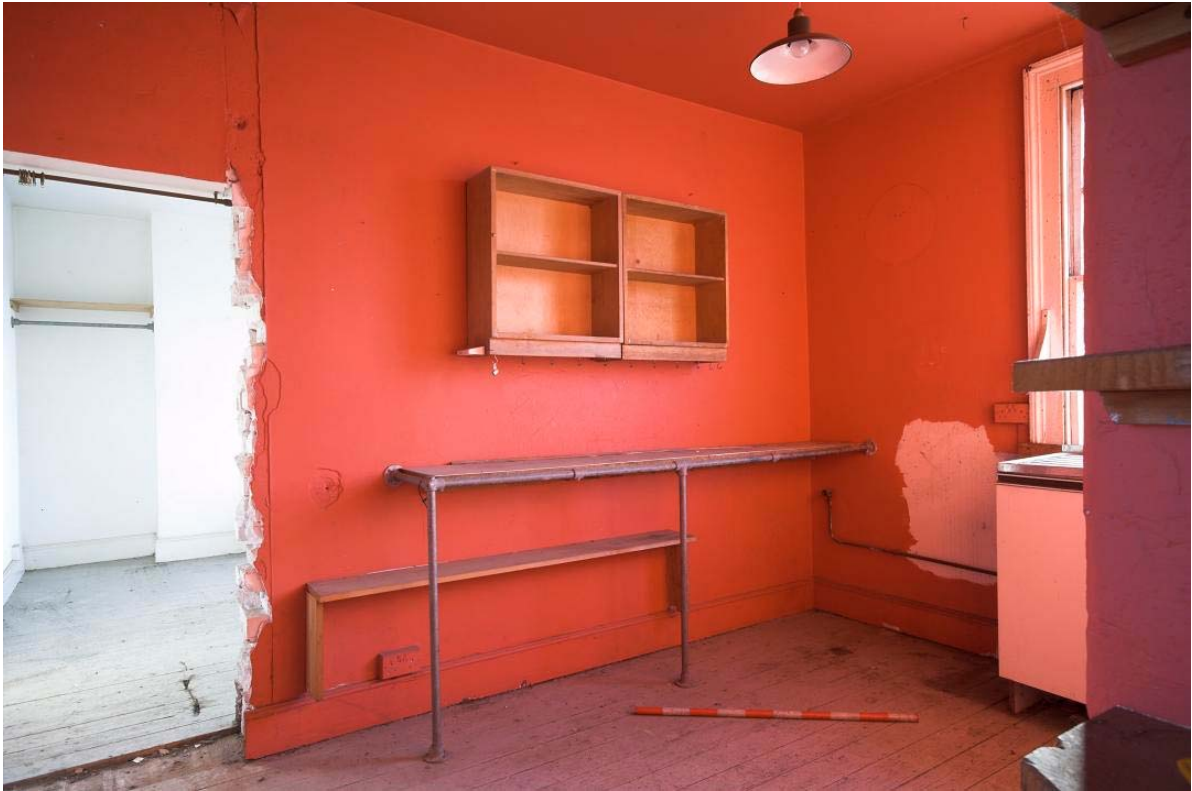
Plate 31: Kitchen CB8C (Figure 17) in Culross Building with window in rear (south-east) wall
