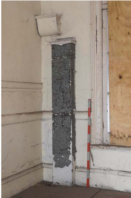
Plate 59: Central heating vent on north-west wall of Room CH1F (Figure 15), Culross Hall
