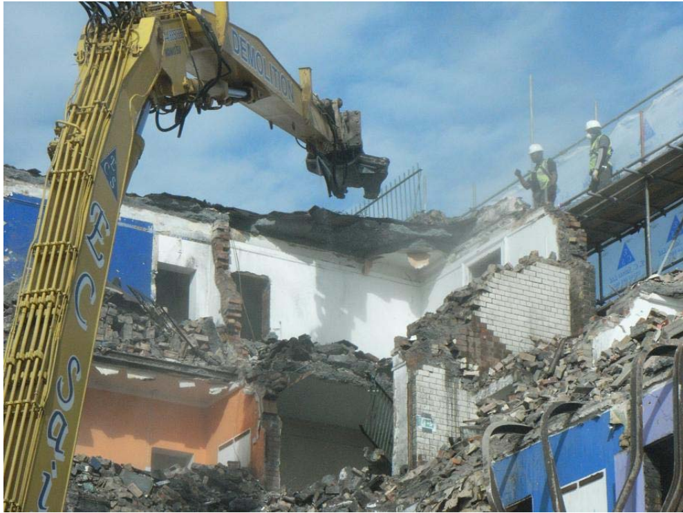
Plate 17: The demolition of the Culross Building showed that its flat roof was formed of screed over concrete
