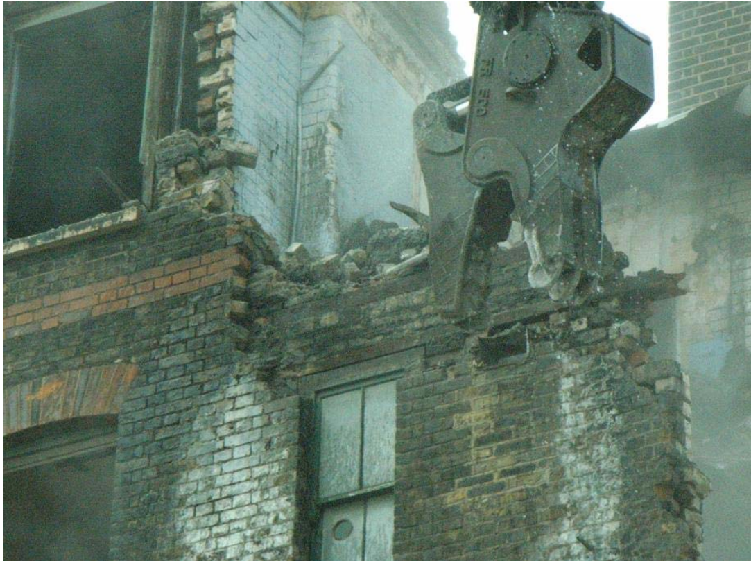
Plate 13: Iron lintel behind window arch in rear (south-east) elevation of Culross Building exposed during demolition
