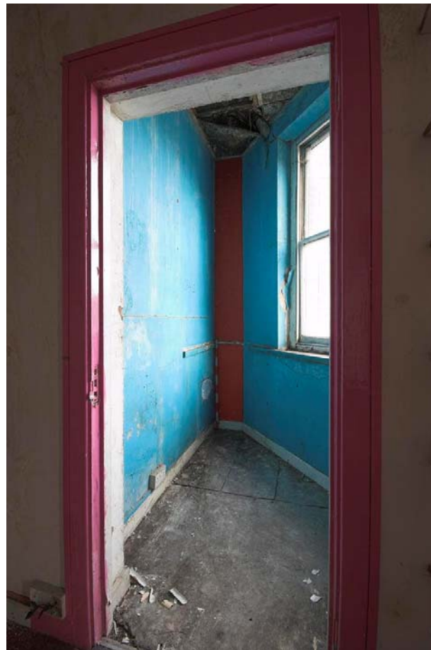
Plate 74: First floor Room CB41I, No. 41 Battle Bridge Road, viewed from the south-west
