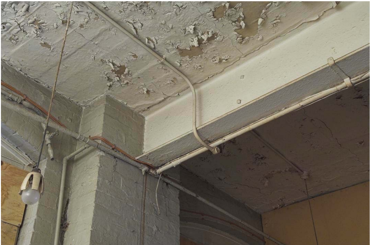
Plate 54: An RSJ supporting the first floor in Room CHGG (Figure 14) in Culross Hall
