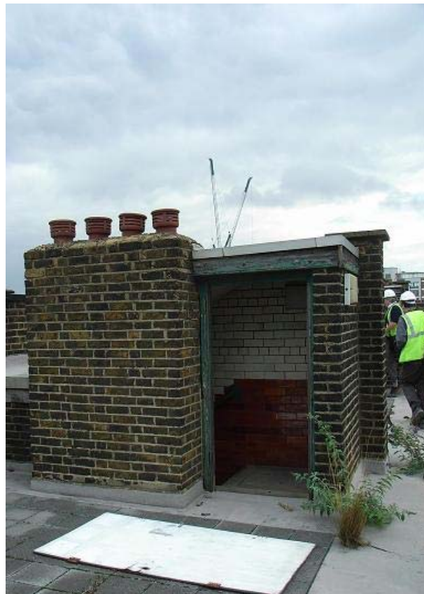
Plate 22: Covered stairway on Culross Building's roof with attached chimney stack (left) and ash chute vent (right), viewed from the south
