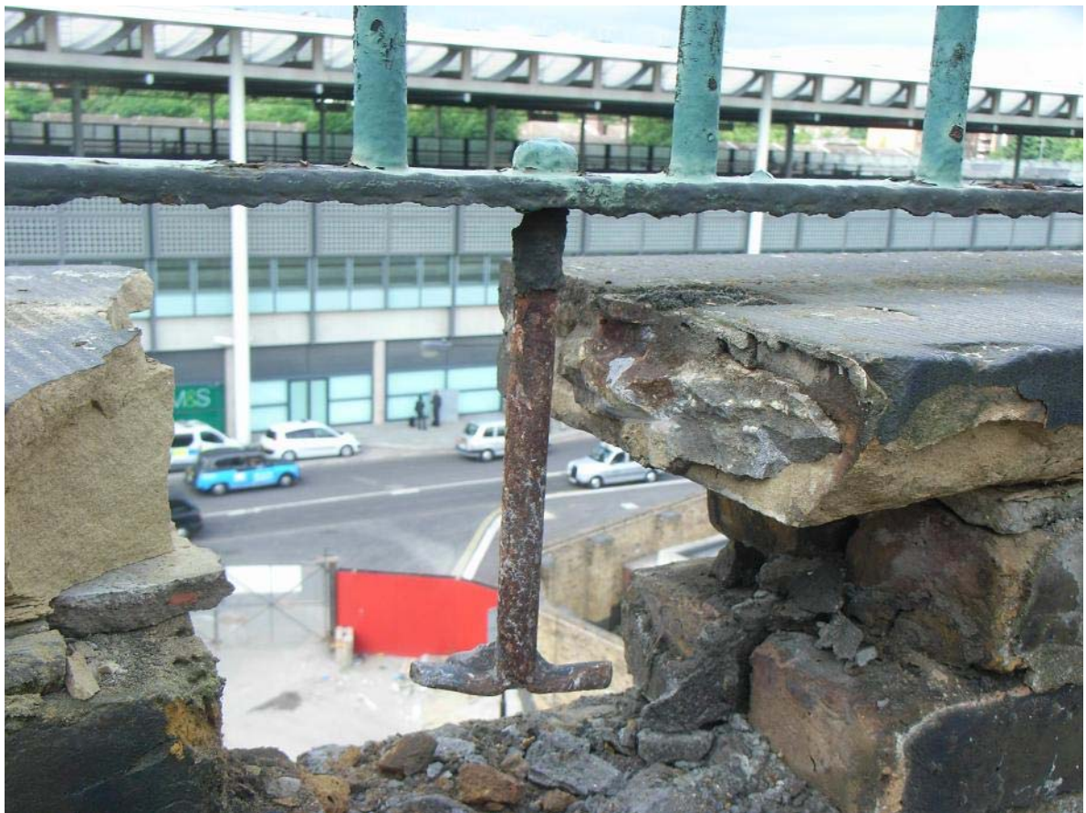
Plate 18: Vertical rod for fastening railing to side (south-west) parapet wall of Culross Building exposed during demolition
