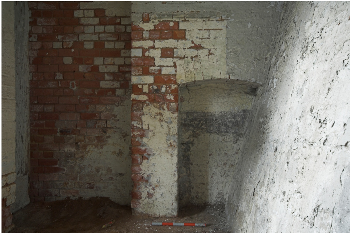
Plate 38: South-west wall of Room CBB2 in the basement below the Culross Building with mass concrete retaining rear wall to the right (north-west)
