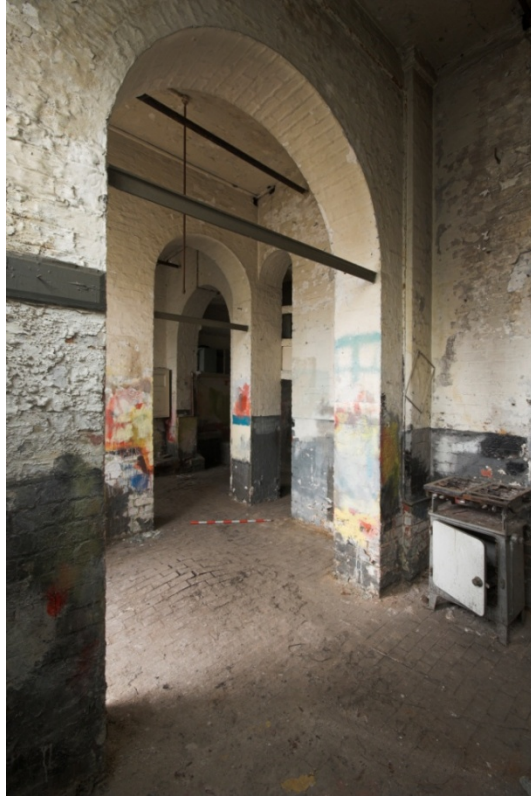
Plate 39: Room CBB9 in the basement below the Culross Building viewed from the east
