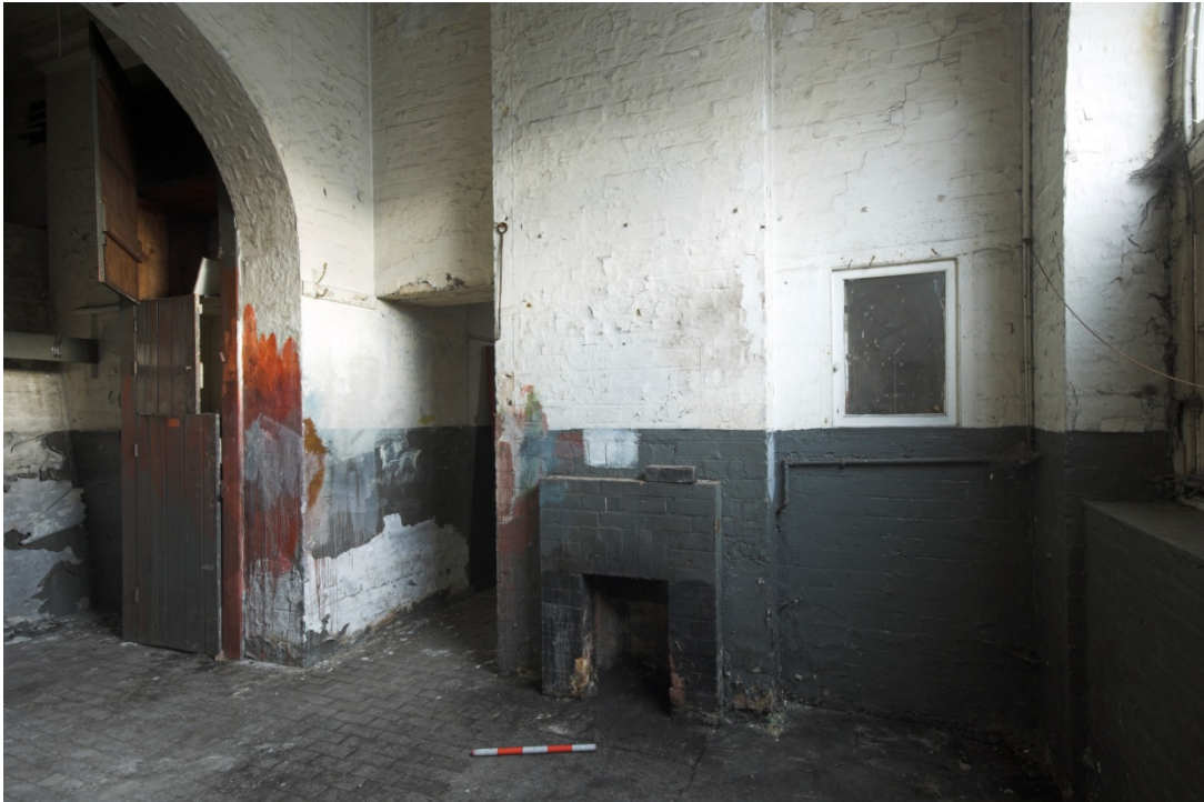
Plate 41: North-east wall of Room CBB13 in the basement below the Culross Building viewed from the south
