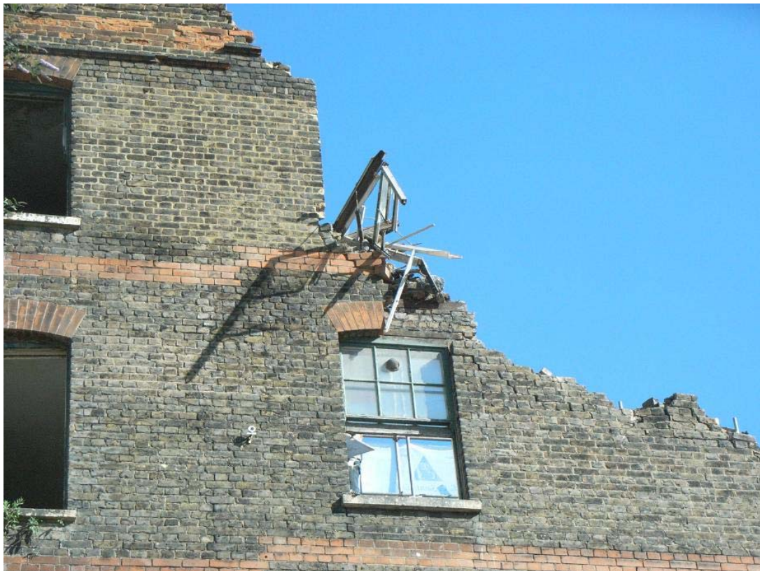
Plate 14: Iron lintel behind window arch in rear (south-east) elevation of Culross Building exposed during demolition
