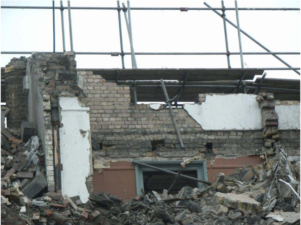
Plate 9: Relieving arch above window on interior (south-east) side of front (north-west) elevation of the Culross Building exposed during demolition
