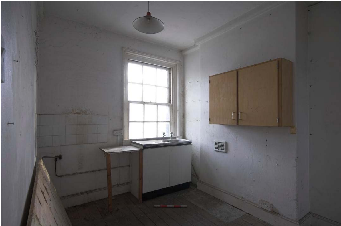
Plate 32: Kitchen CB6C (Figure 16) in Culross Building with window in rear (south-east) wall
