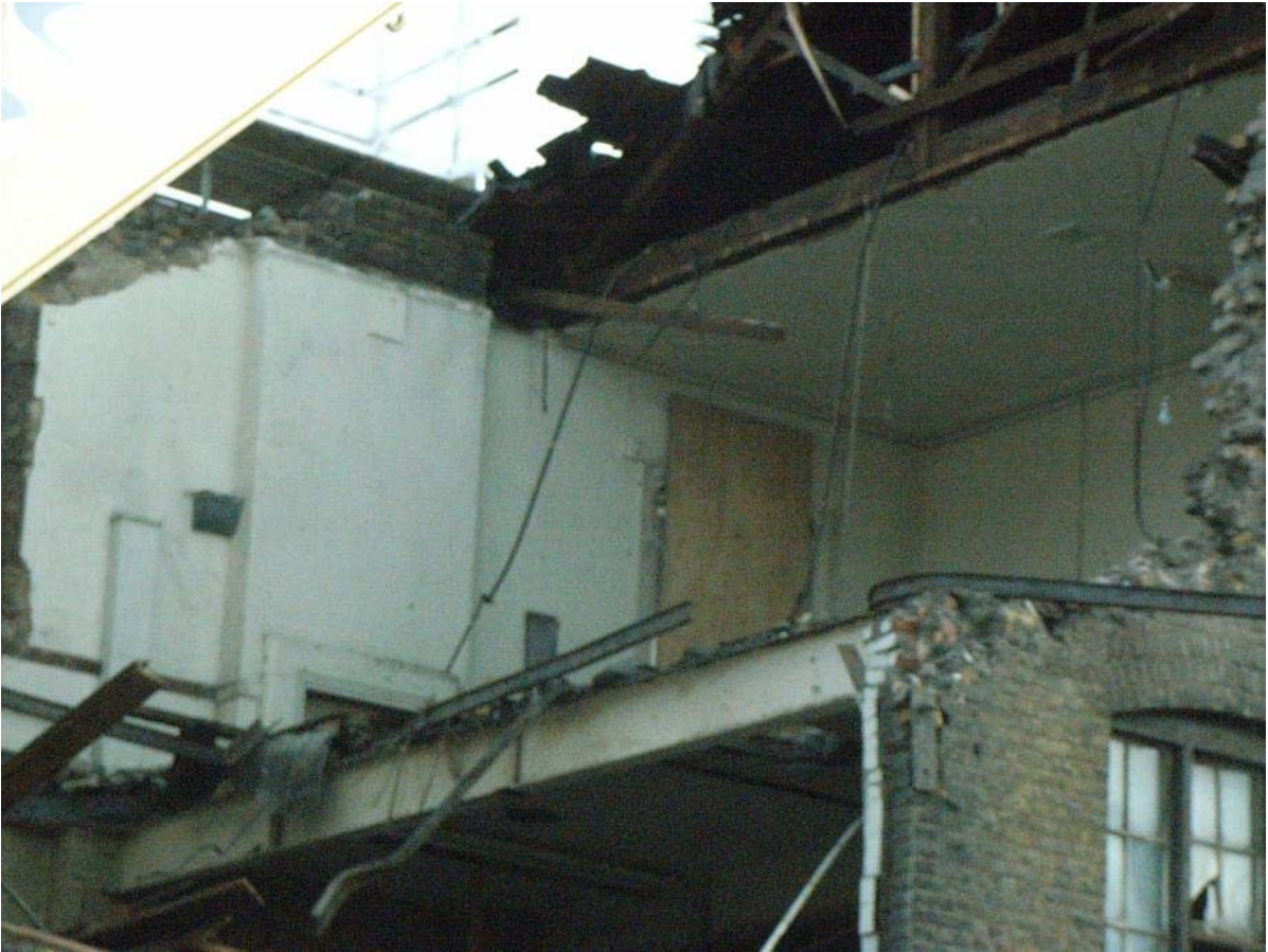
Plate 55: Room CH1F (Figure 15) on first floor of Culross Hall looking north during demolition
