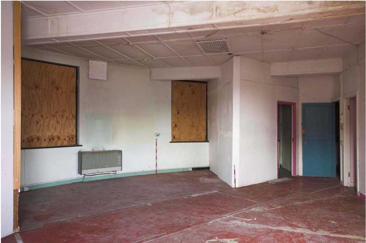
Plate 73: First floor Meeting Room CB41L, No. 41 Battle Bridge Road, viewed from the south
