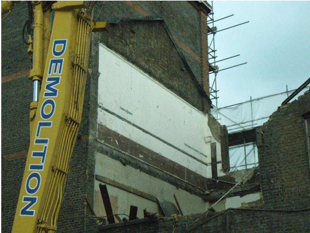
Plate 43: Straight joint between Culross Hall (right) and Culross Building (left) on the rear (south-east) side of the buildings during demolition
