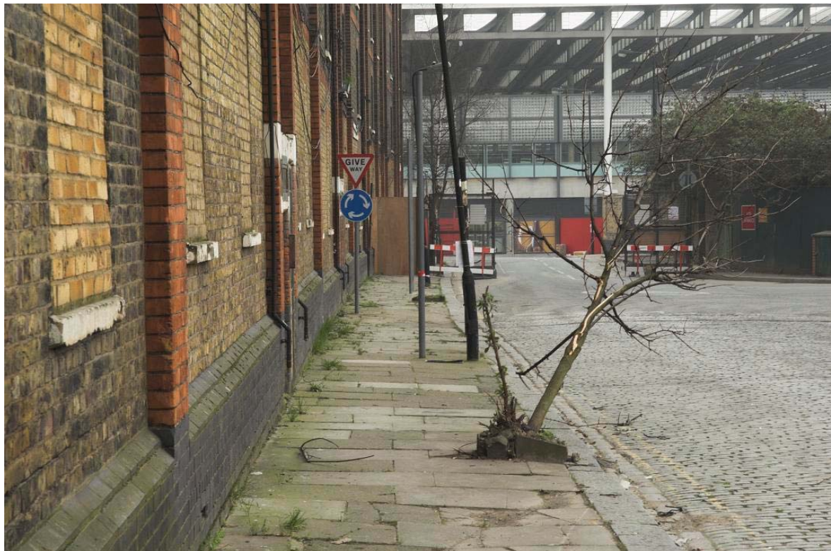
Plate 8: Brick plinth on front (north-west) elevation of Culross Building (viewed from the north-east)
