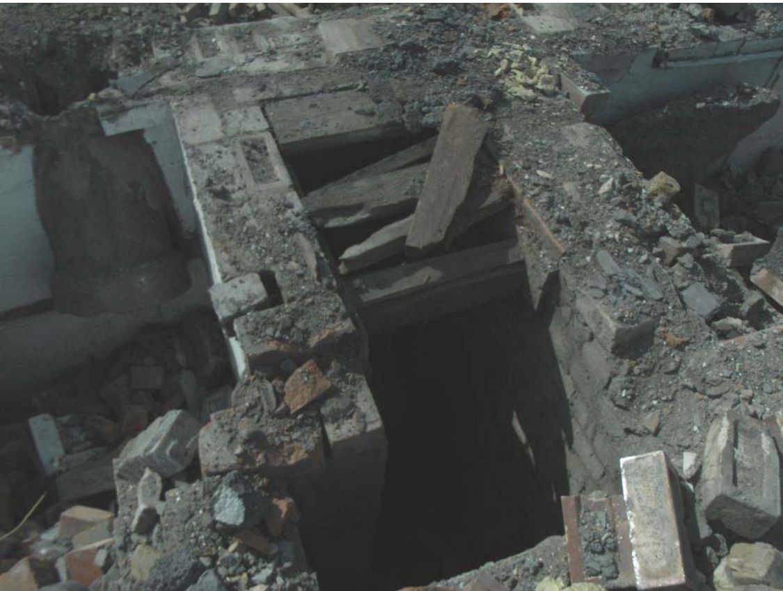
Plate 28: Foot of ash chute and void beneath stairwell to Culross Building Flats 1 to 8
