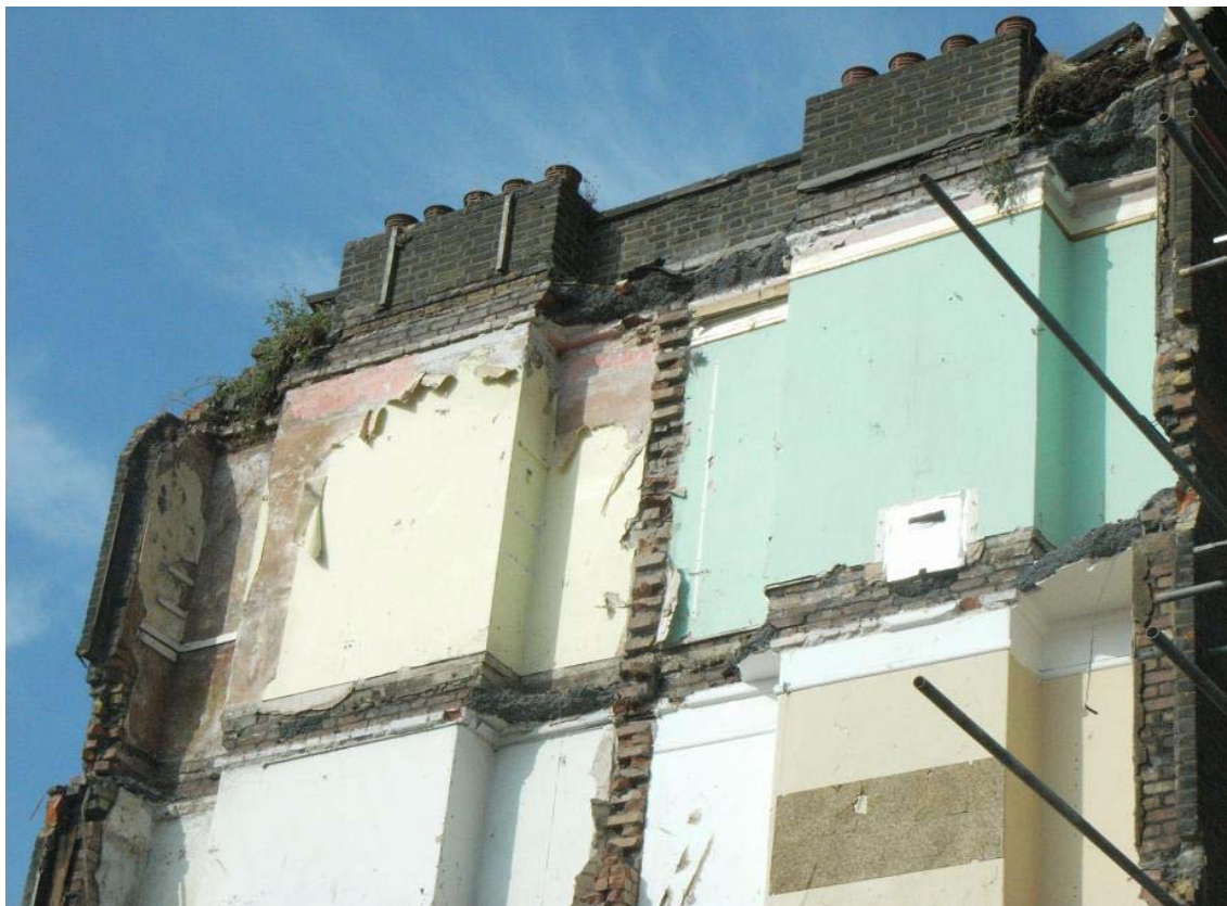
Plate 20: Dividing wall between Culcross Building flats (viewed from the south) exposed during demolition
