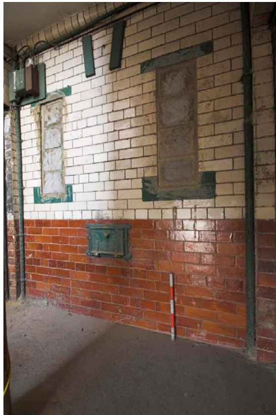
Plate 26: Blocked windows and ash chute in stairwell between Flats 5 and 6 (Figure 16) of Culross Building
