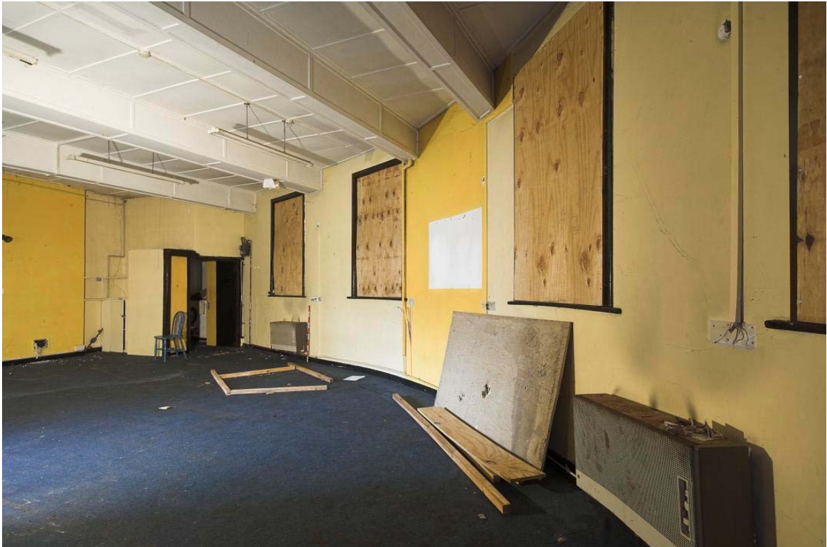
Plate 72: Covered RSJs in ground floor Meeting Room CB41D, No. 41 Battle Bridge Road, viewed from the north
