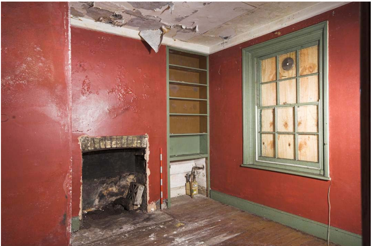
Plate 36: Living Room CB18D (Figure 14) in Culross Building with window in front (north-west) wall
