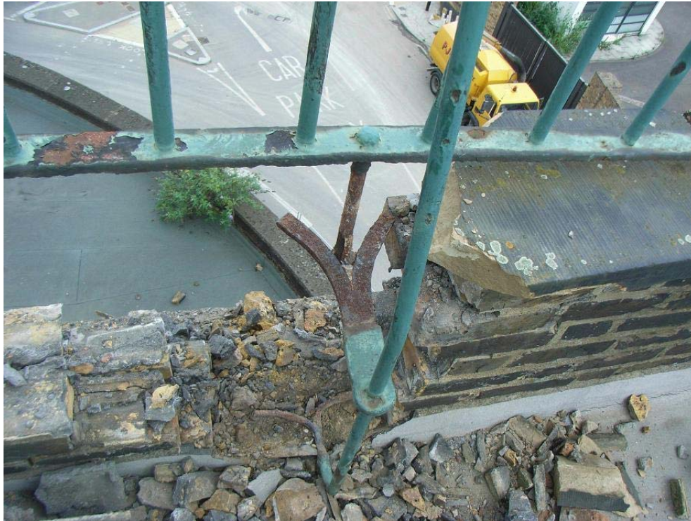
Plate 19: Horizontal fastening for railing on side (south-west) parapet wall of Culcross Building exposed during demolition
