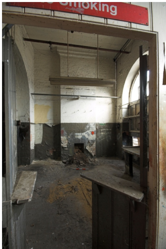
Plate 40: North-east wall of Room CBB7 in the basement below the Culross Building viewed from the south-west
