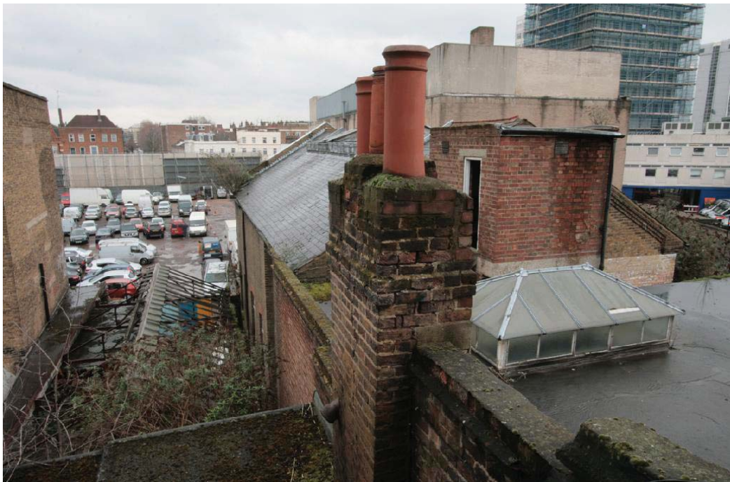
Plate 12. View looking southeast of theatre and flat roof to rear of 11-12 Paddington Green.
