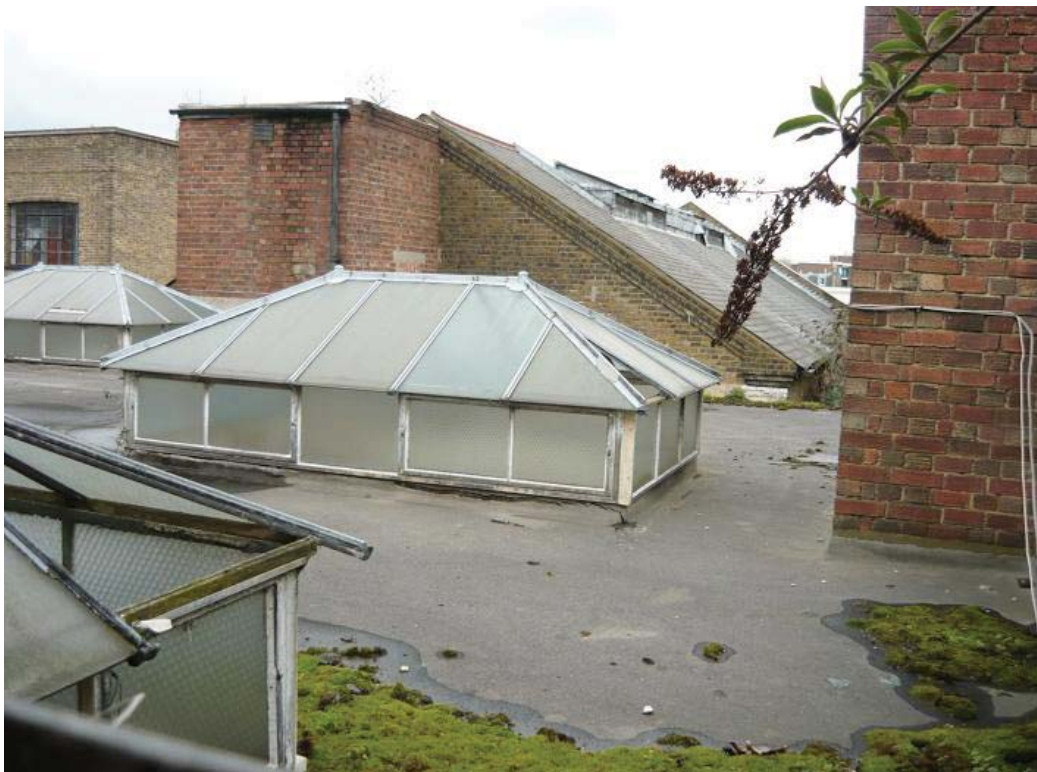
Plate 13. Skylight and flat roof over first floor of 11-12 Paddington Green, with gable end wall of theatre beyond showing added red brick lift shaft and scar from previous roof structure.
