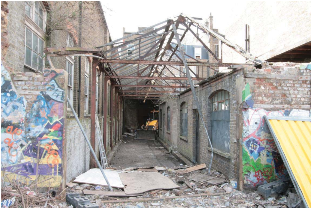
Plate 6. Derelict canopy over rear yard of 13 Paddington Green, theatre windows visible on left.
