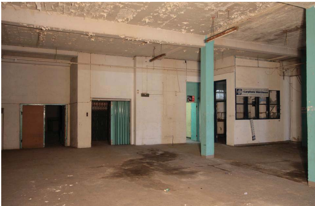
Plate 16. Ground floor of 11-12 Paddington Green, looking east, with entrance to theatre on left.
