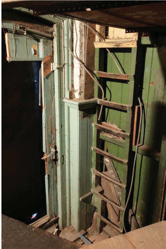
Plate 21. Ladder to intermediate floor level in wings, tongue and groove panelling and arched exit door to south elevation of theatre, view from the stage.
