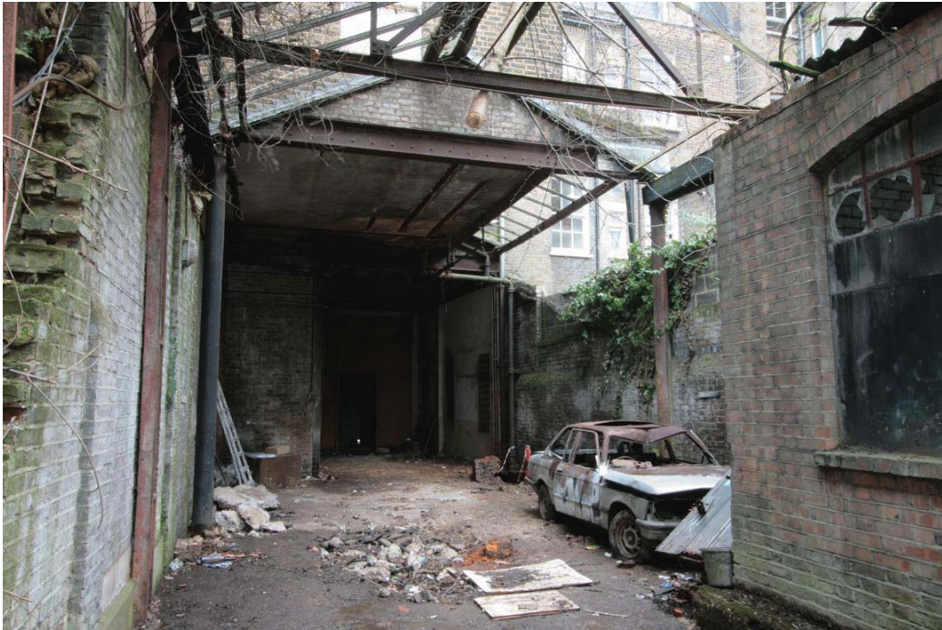
Plate 7. East/rear elevation of 13 Paddington Green, blocked gateway to street beyond and projecting first floor.
