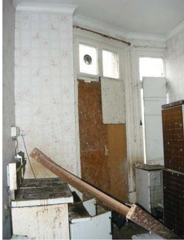
Plate 37. First floor room F2, full height original windows and partition wall on right.
