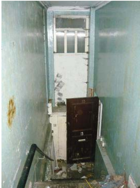
Plate 35. 13 Paddington Green entrance hall showing relocated front door and inserted steps up to ground floor level, the original floor level can be seen on the wall.
