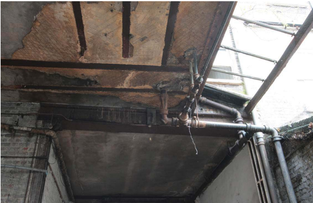
Plate 8. Detail view of underside of projecting first floor of 13 Paddington Green.
