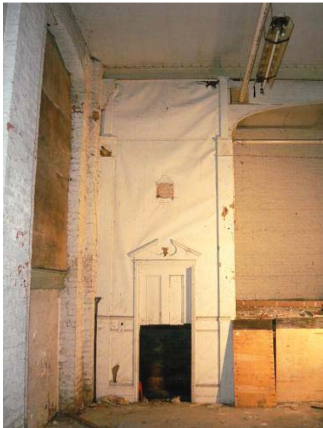
Plate 18. Detail of timber stage façade and door to under stage room, visible on the left is a shadow and scar where tongue and groove panelling once ran the length of the side wall.
