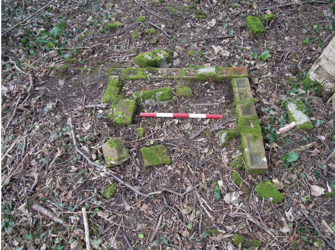
Plate XVII , Brick base or man-hole on south-west side of lower terrace F. 9 (scale, 50 cm)
