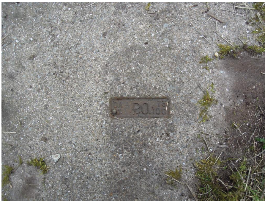
Plate X , Detail of concrete cover of inspection chamber F.1, showing iron 'P O' plaque
