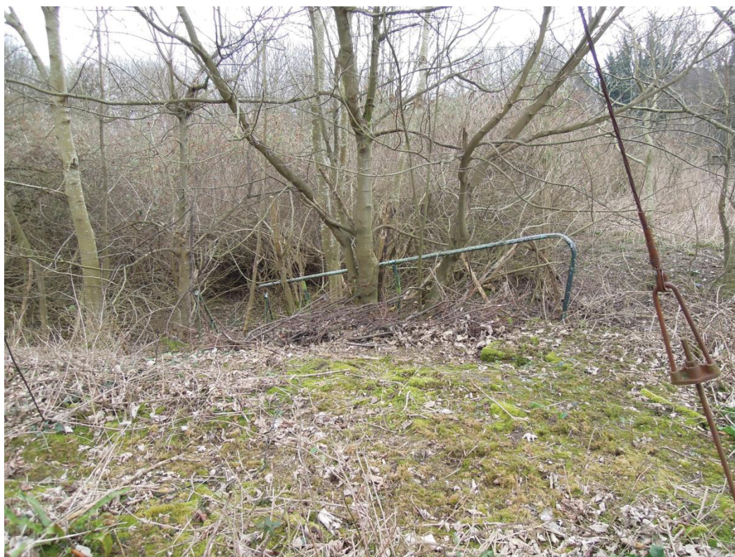
Plate XIII , General view of steps and hand-rail F. 7 leading down from marshalling yard, looking south-east
