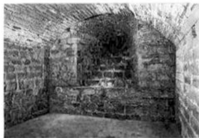
Fig 77 The twelfth century window embrasure in the south wall of the ground floor (room 1) (photo: Carlisle Archaeological Unit)
