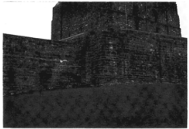
Fig 33 The re-entrant, showing the rise in ground level on the berm of the outer ditch at this point (photo: Carlisle Archaeological Unit)
