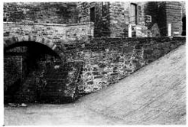
Fig 60 The north side of the inner bridge and buttresses from the inner ditch (photo: Carlisle Archaeological Unit)
