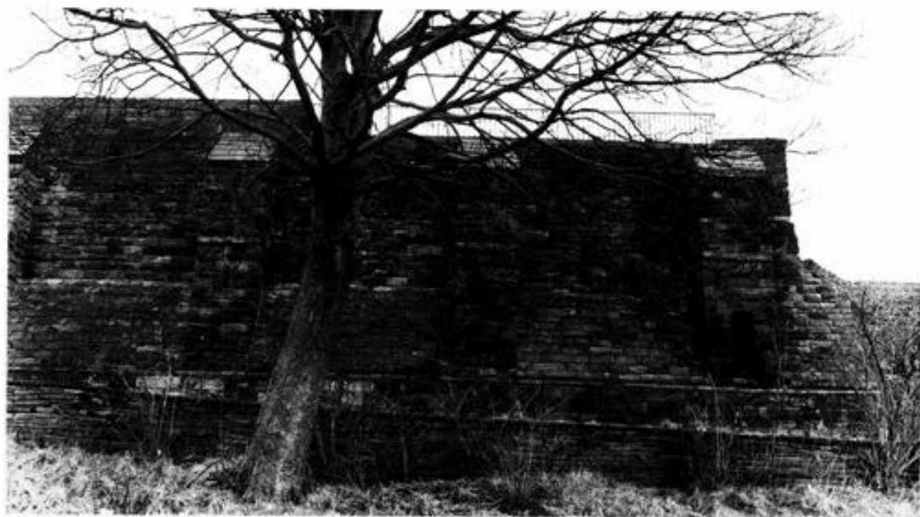
Fig 28 The west curtain wall at the south-west corner; this may be part of the wall documented in 1318–21 (photo: Institute Advanced Architectural Studies, University of York)
