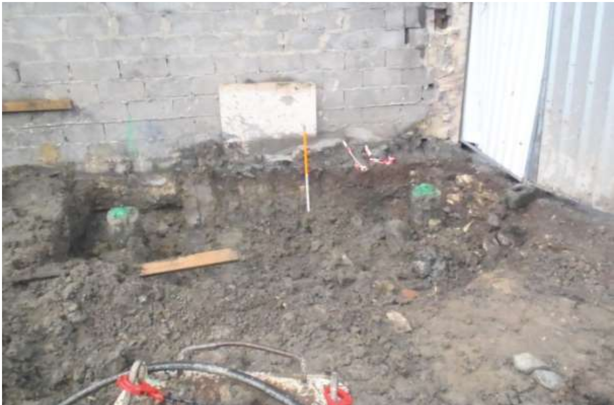
Plate 1 South end of site showing excavation around piles to form concrete ring beam.
