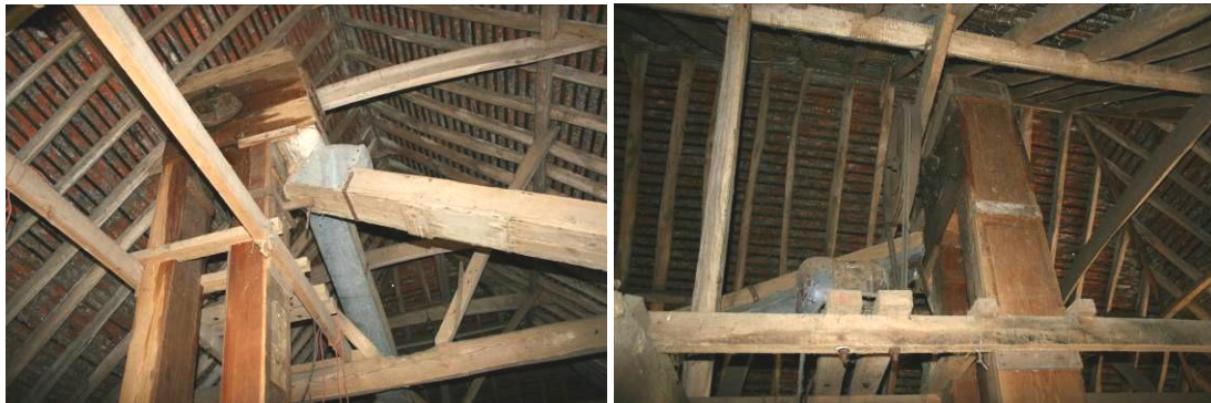
The head of the elevator with its two grain slides. The electric motor drives the belt elevator.
