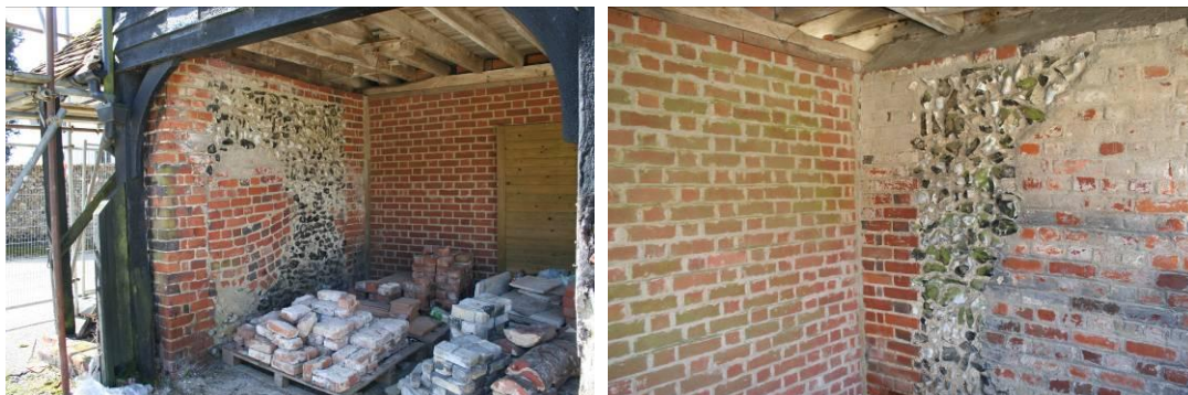
The internal surfaces of the end lower walls. Both have been rebuilt in the C19th.
