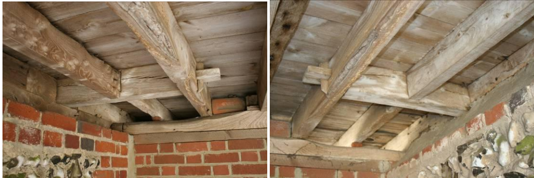
The cantilever supports for the lucam. East (left) and west sides of the building.
