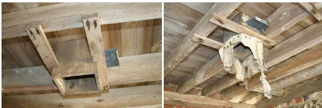
Chutes to empty the grain bins.
