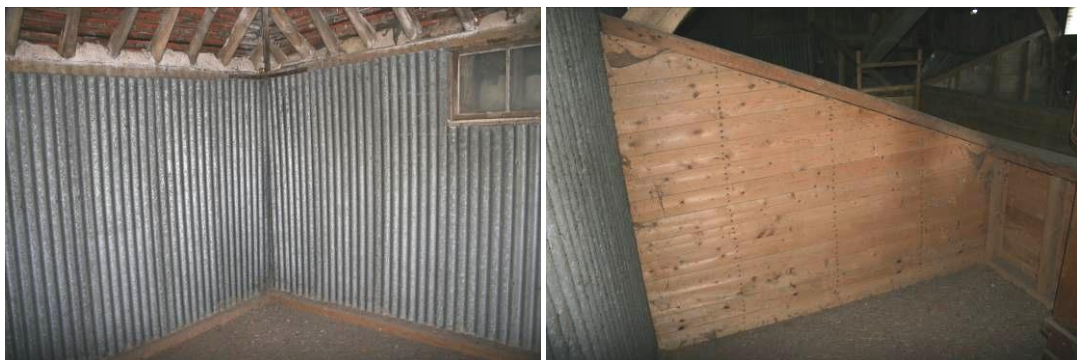
The NW corner and western central bay are clad with corrugated iron sheets.
