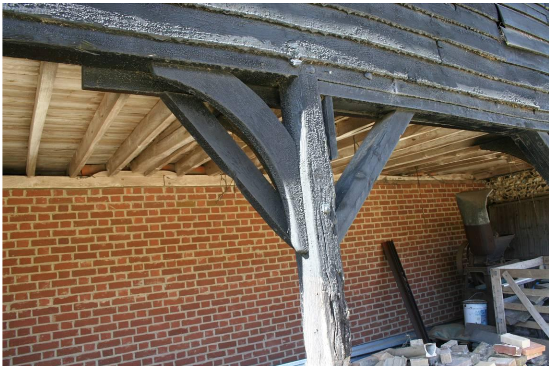
Support post showing original curved brace and later repairs.
