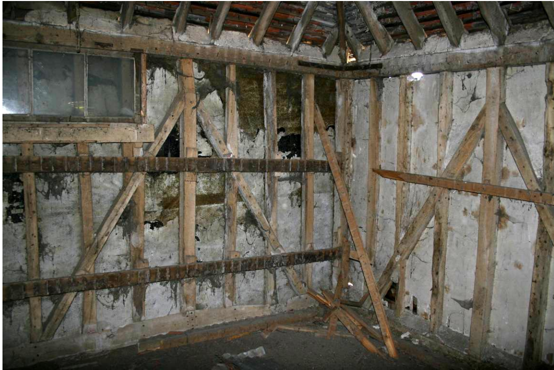
The NE corner of the granary showing the scantling frame and plasterwork.
