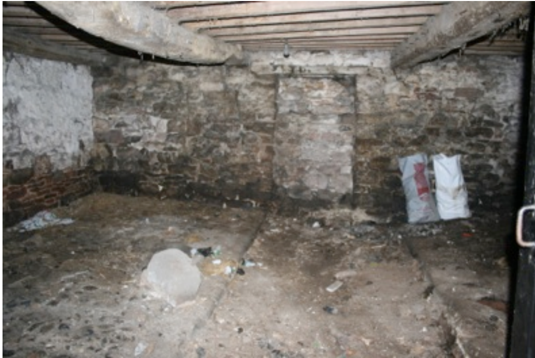
Plate 3. Inside of Byre Showing Cobbled Floor, Central Passage and Blocked up Door.
