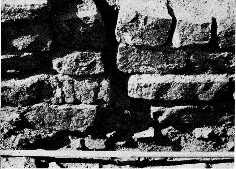
PLATE III.—Turret east wall, settlement crack.
