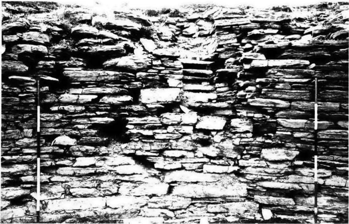
ILL. 13 : The inner face of the broch wall on its N side: some of the cavities may be explained by the subsequent disintegration of the sandstone used in the construction. Part of the stone ladder is visible
