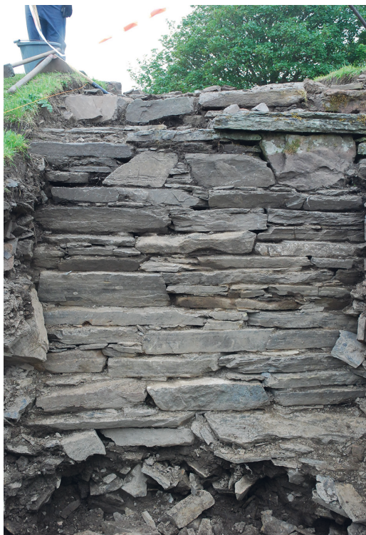
ILLUS 2 The infilled gully beneath Thrumster broch: a rare example of prepared foundations for a broch wall
