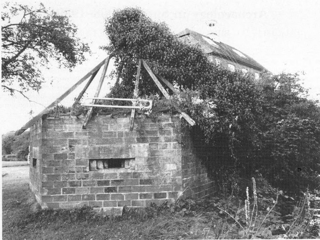
Fig 1. Elstead Mill, SU 903 438: pillbox originally disguised as a summer house. Photograph by C Shepheard
