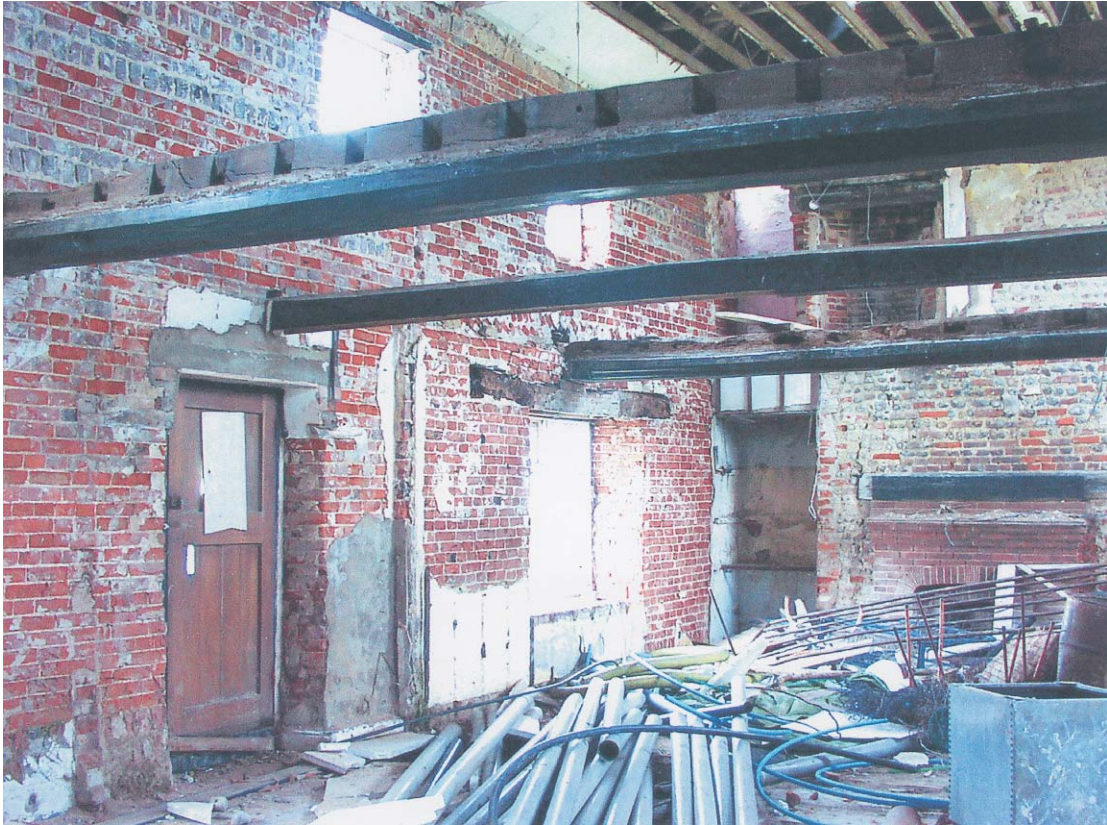
Plate 10 The increase in thickness of the ground floor west wall that starts 0.66m away from the door
