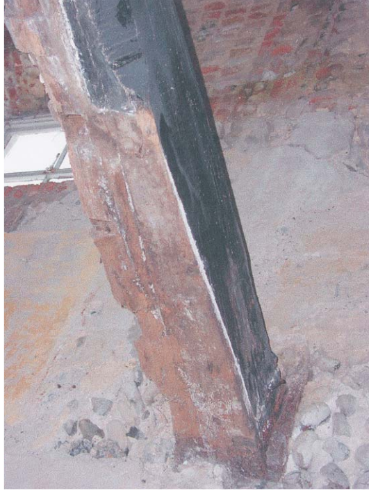
Plate 5 Position of stairs on 17th-century beam as indicated by the position of the chamfer stop
