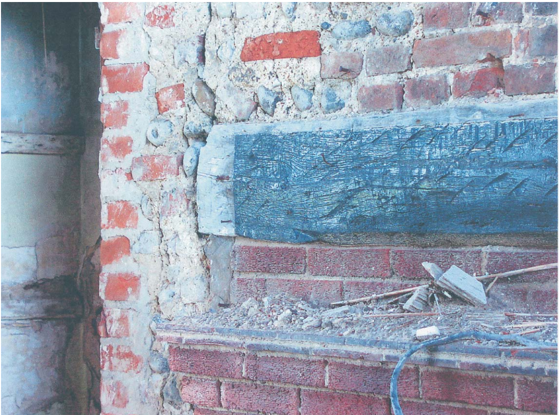
Plate 7 Chamfer stop associated with the north stack fireplace at ground floor level
