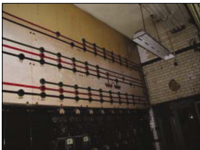
Plate 45: The Electric Lighting Station Gatehouse, Detail of Supply Board
