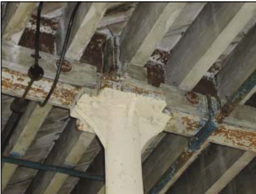
Plate 21: The Star Brush Works, Detail of Column and Joist Bracing from 2nd to 3rd floor
