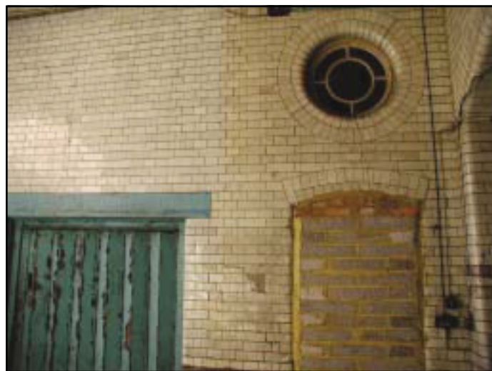
Plate 32: The Electric Lighting Station Gatehouse, Detail of Side Entrance and Oriel Window
