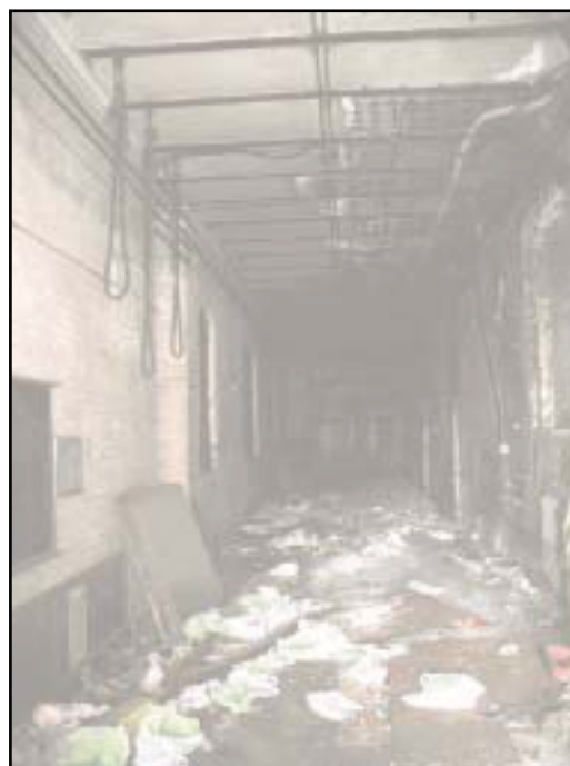
Plate 34: The Electric Lighting Station Gatehouse, Blocked Access Way to Demolished Power Station
