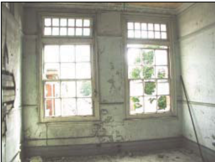
Plate 37: The Electric Lighting Station Gatehouse, Interior View of 1st Floor Facade Windows
