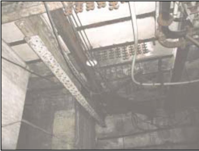
Plate 35: The Electric Lighting Station Gatehouse, Detail of Roof Support and Cable Ducting
