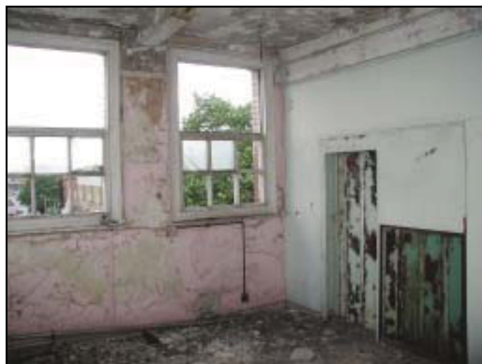
Plate 44: The Electric Lighting Station Gatehouse, 2nd Floor Front Room Front Window and Inserted Lift.
