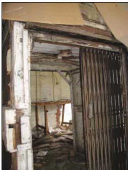
Plate 23: The Star Brush Works, Ground Floor Goods Lift
