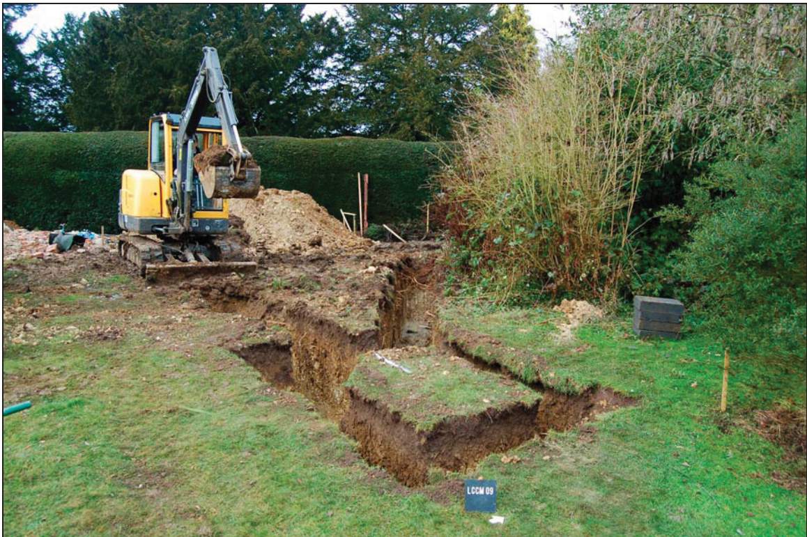
Plate 2 Excavation for pool house on undisturbed ground to the east of the moat
