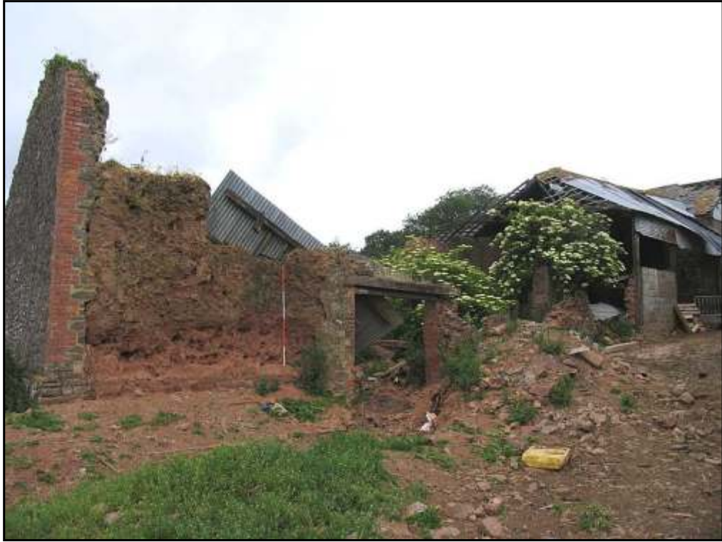
Plate 7 Root house and cattle shed, showing first floor level jamb in the cob walling.
