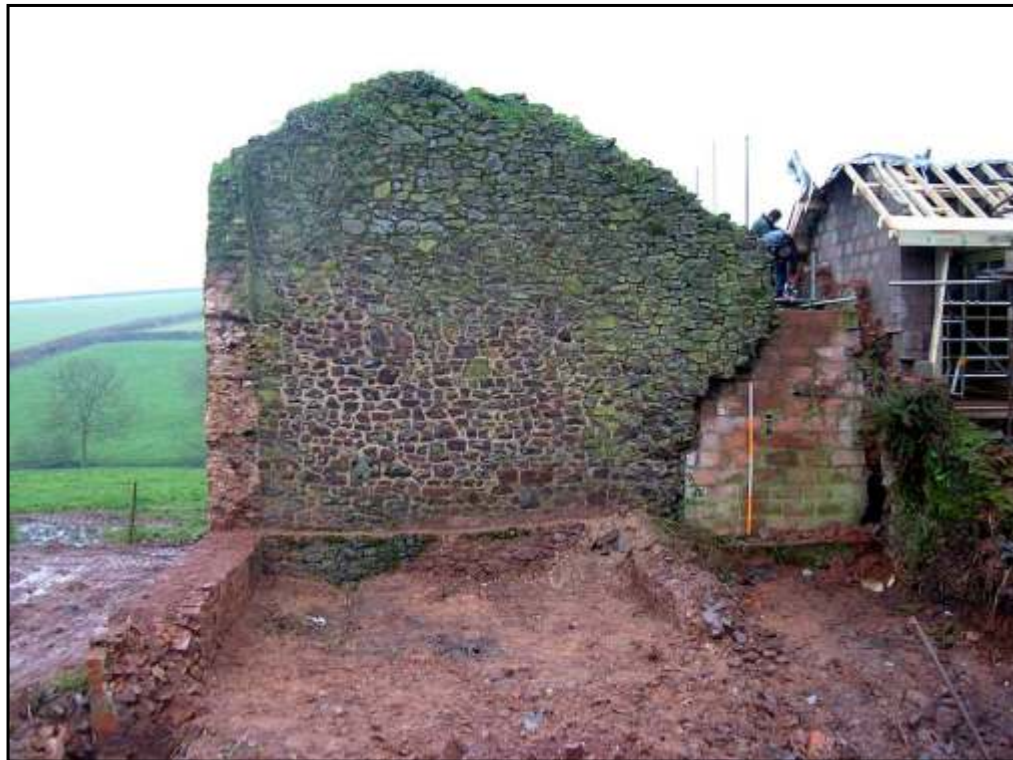
Plate 8 The southern end of the root house after removal of the rubble and demolition of the cob walling.
