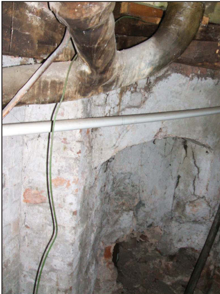
Plate 2 Ground-floor store behind the stairs showing arch and 'splayed' masonry, looking east.
