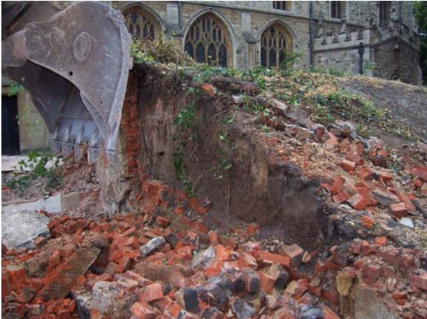
Plate 1: Area 2, during the removal of the earth mound and associated late 19 th century wall
