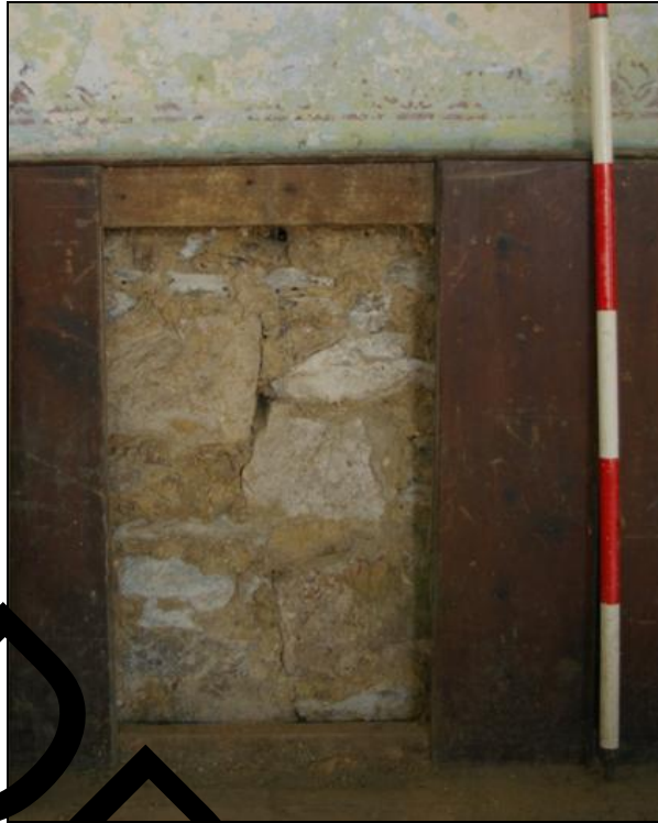
Figure 12: The interior face and fabric of the east wall, exposed where panels have been removed; viewed from the west.
