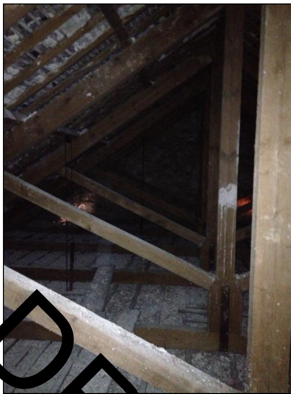
Figure 19: The kingpost roof trusses on the east pitch of the chapel, viewed from the north.
