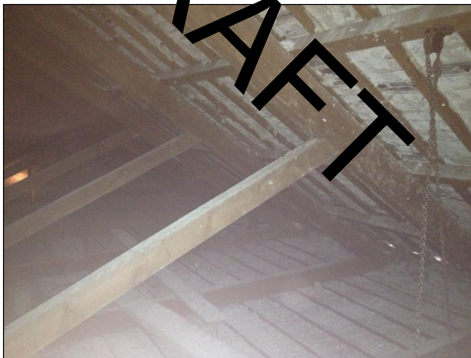
Figure 20: The truss blades, purlins and struts on the west pitch of the roof, viewed from the north.
