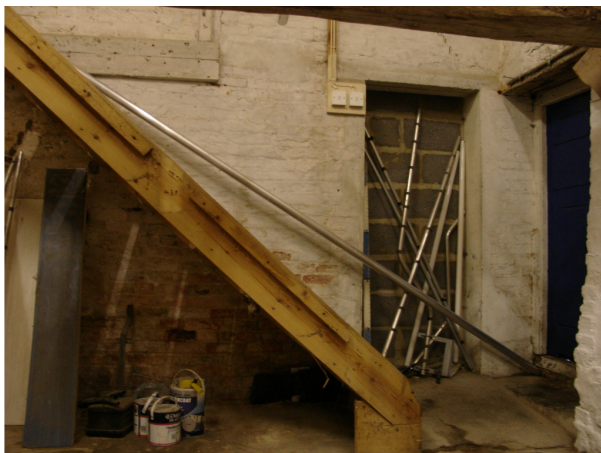
Plate 10 View of southern storeroom interior showing staircase to first floor, access door to room and blocked doorway in south elevation, looking south
