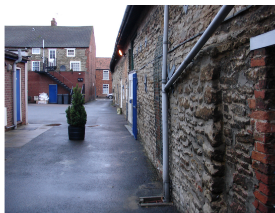
Plate 4 General view of surveyed building and electrical store yard, Boston Road at rear of photograph, looking north
