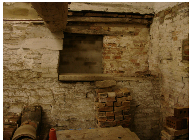
Plate 11 View of southern storeroom interior showing alcove at southwest corner of room, blocked opening and brick and wood insertion under beam '1' in east wall and blocked joist holes and opening in south elevation, looking east
