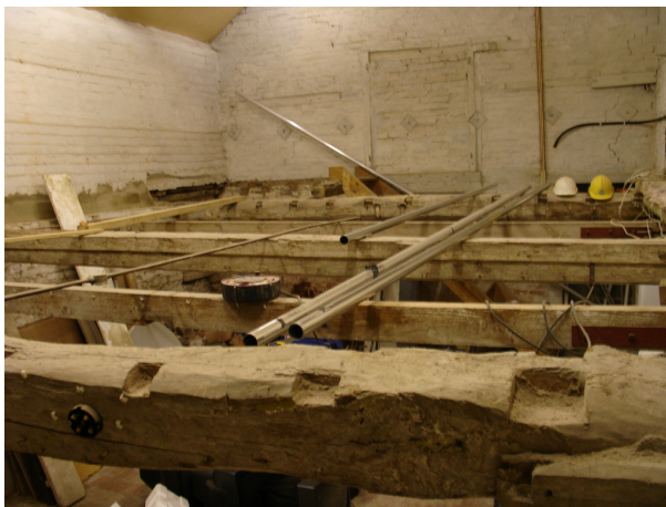
Plate 9 View of southern storeroom interior showing first floor beams '1-5' and south elevation, including blocked entry and tension bolts, looking south
