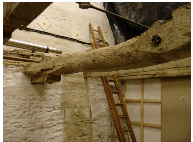
Plate 12 Southern storeroom interior showing detail of possible original beam '5', looking northwest. Partition wall to workshop and storeroom at right, access to first floor store via ladder
