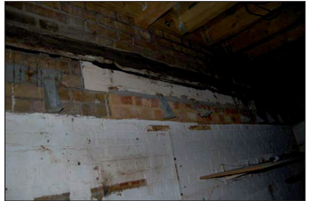
Plate 26: Room G10: lintel over bricked up window to G3
