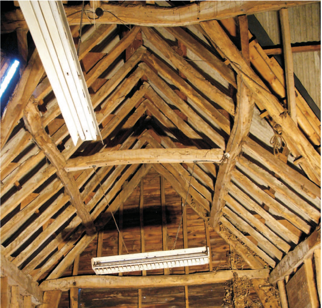
View into mid-strey roof, built a single bay unit with purlins framed front and rear and birds mouth collar between. Purlins converted from one tree sawn through the centre. These again suggest possible coppice growth pattern.
