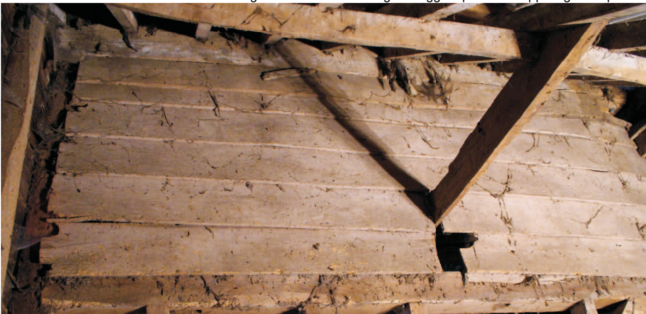
Possible original elm weatherboarding trapped by the lean-to roof. Still in good condition.
