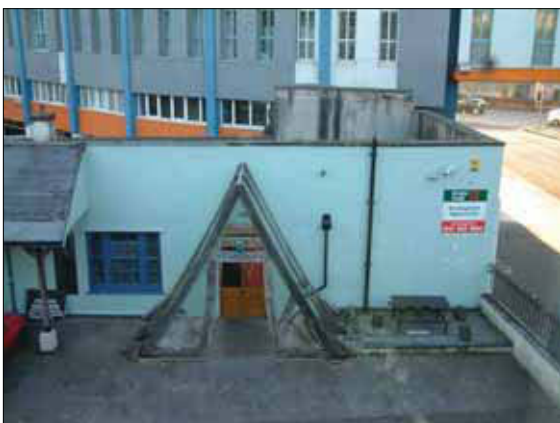
Plate 7: view of the southwest end of the Attic Bar and Nightclub showing the earlier masonry remnant with unfinished eastern side forming the higher section of parapet wall, looking southeast from an attic room in the Full Moon Hotel opposite
