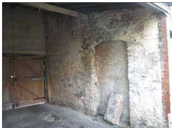
Plate 12: bricked-up doorway and adjacent small window preserved in the remnant masonry wall defining the south side of the Wilder Street entrance, looking east
