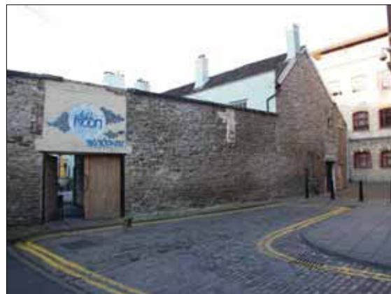
Plate 10: Wilder Street entrance sealed with double timber doors set in the masonry wall defining the site boundary and rear of the hotel, looking west
