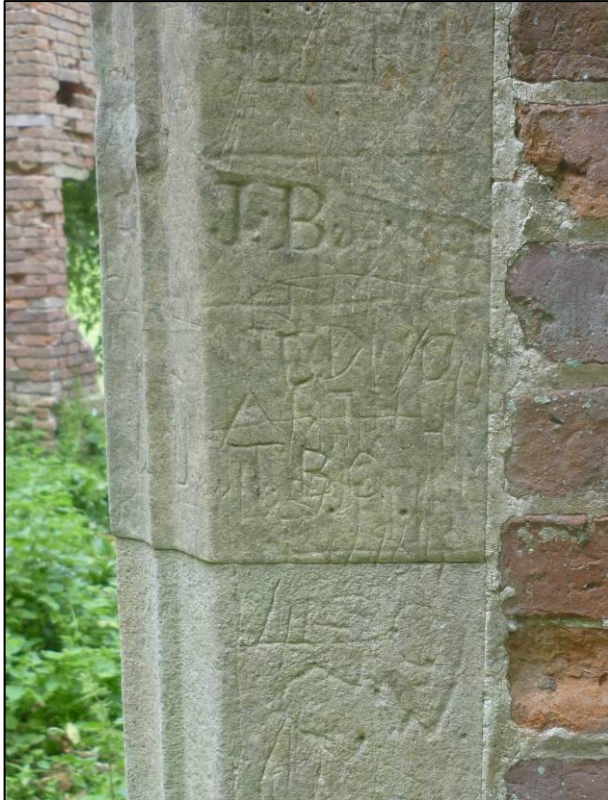
Plate 8: Graffiti on external north jamb of Side C (photo 3/373).
