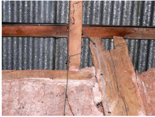
Head of post in north-west corner, with later roof truss principal to left
