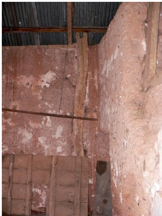
Post set in cob wall in north-west corner. Displaced central door to bottom left
