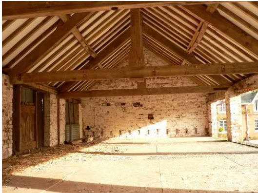
Tallet floor, looking east. Note joist holes in wall above present floor level
