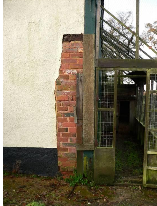
Brickwork repair at north-east corner of barn, with corrugated cladding to north gable
