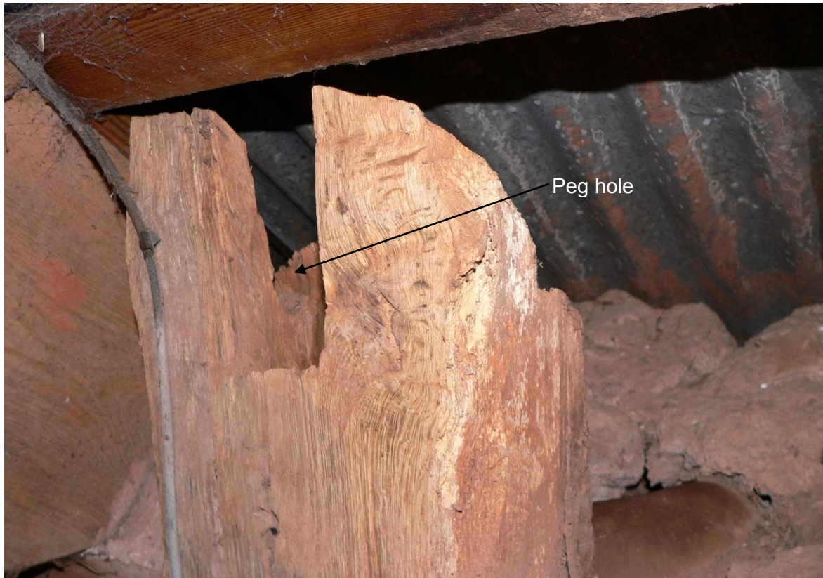
Detail of head of north post, showing mortise and remains of peg hole on left side
