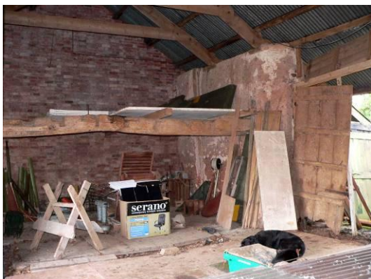
Looking to south-west corner, showing beam formerly carrying first floor at south end and west central doorway
