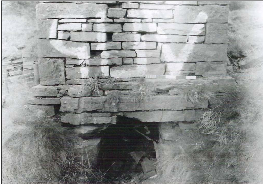
Plate 5: Flue at Base of East Elevation
