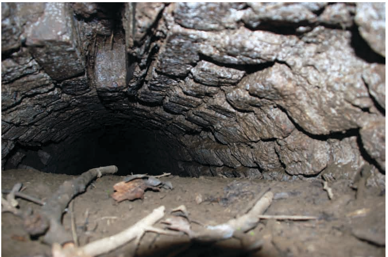
Plate 10 View along the disused flood arch, showing its hand-made brick vault, looking northwest.
