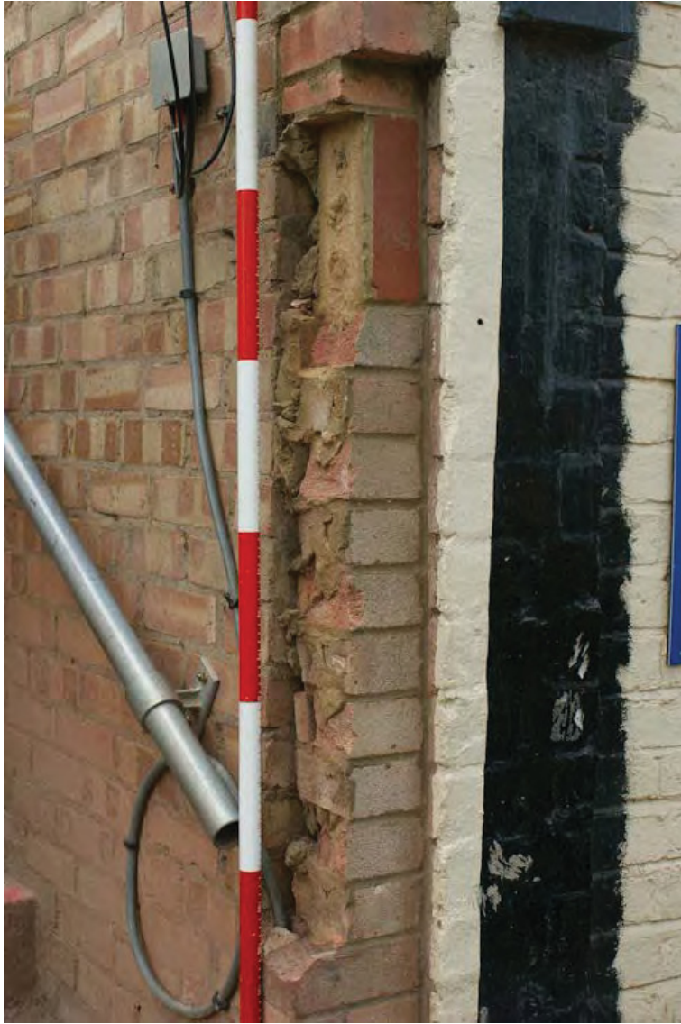
Plate 10: Detail of the building break to the south elevation of the building
