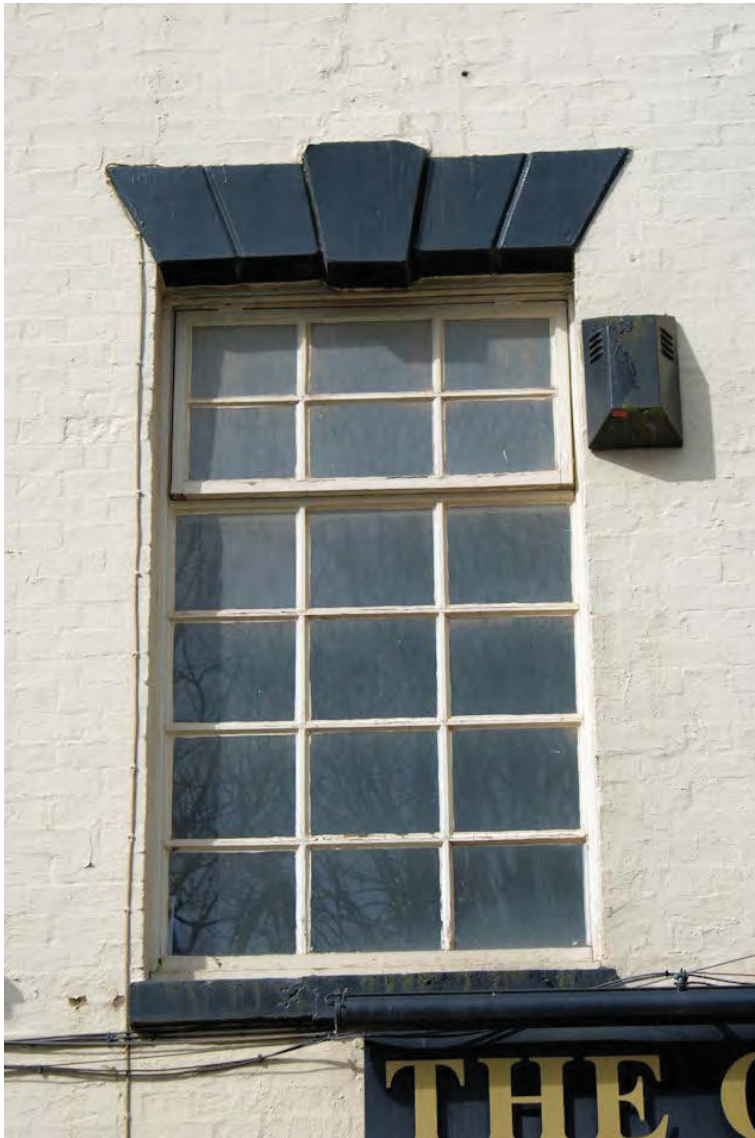
Plate 2: Detail of a first floor window opening, including rusticated arch with keystone
