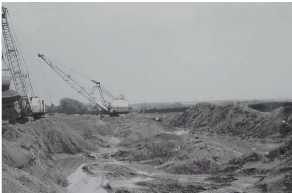
Figure 1.14. Gravel extraction at Chainbridge Lane, Lound, Nottinghamshire in the late 1980s. (Source: © Jen Eccles).
