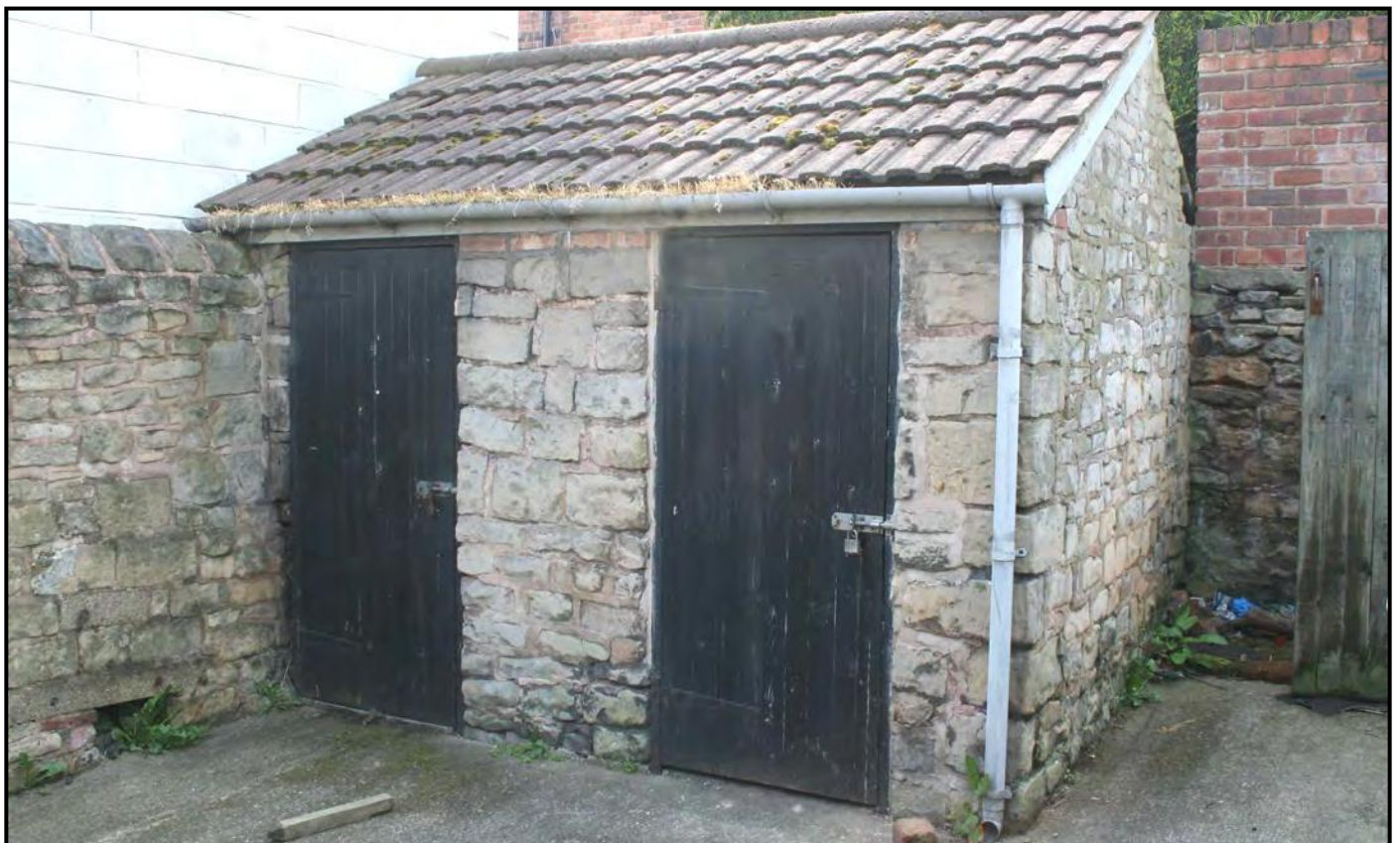
Fig. 59 An original stone-built two-compartment outhouse situated behind Stone Row, dating to before 1875.
