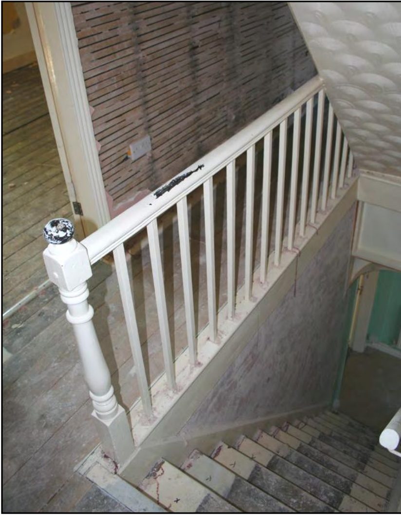
Fig. 13 Internal view of one of the houses at New Bolsover, showing a staircase and part of a stripped lath and plaster partition wall at first floor level.
