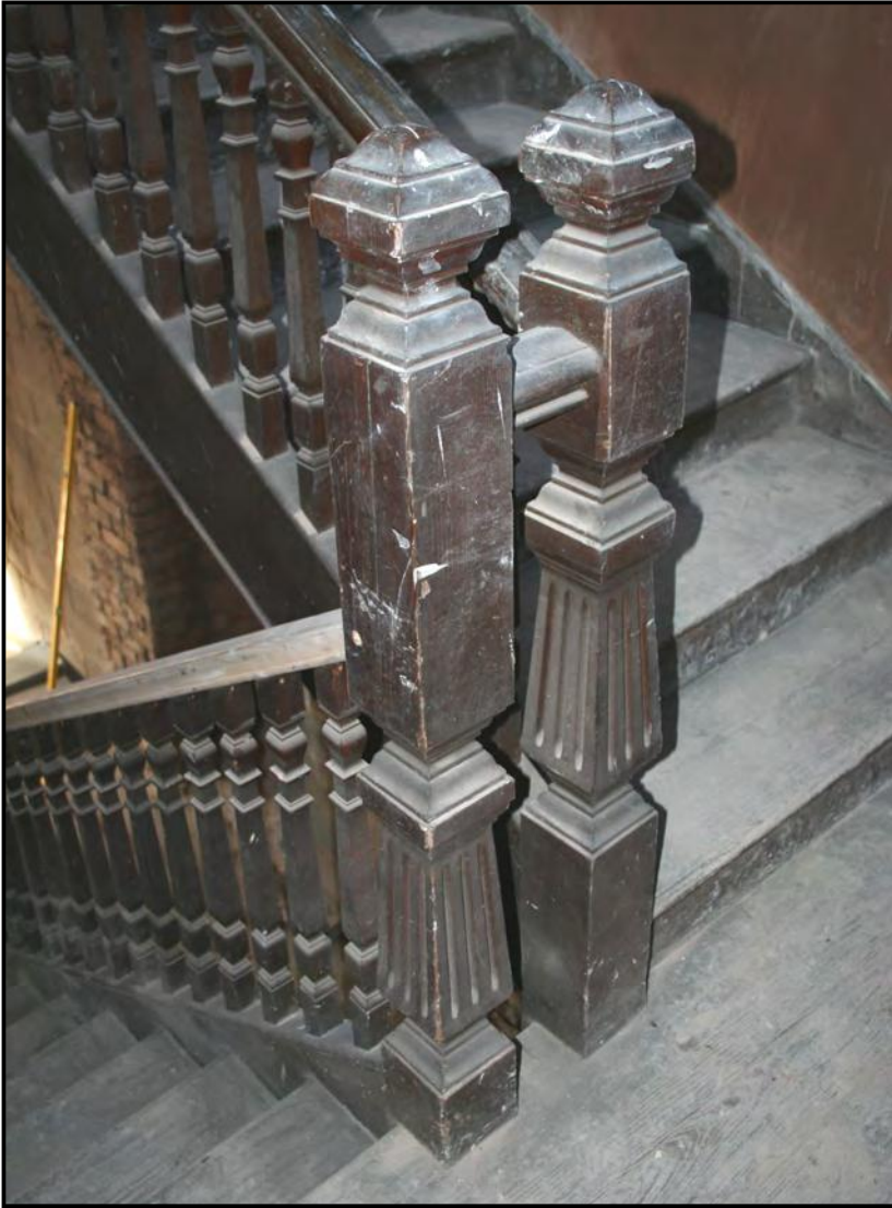
Fig. 23 Detail of the original Victorian staircase remaining in the former stores building at New Bolsover.
