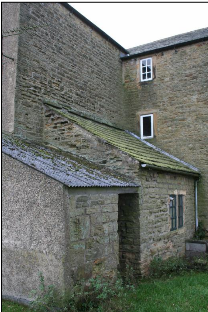
Plate 8: Thin-coursed 18th century stonework showing at the join of the west and south wings of the L-shaped building. The original dairy is the lean-to in the middle.
