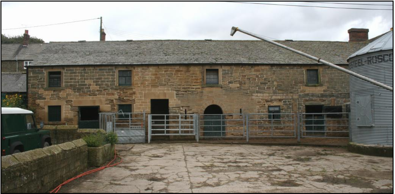
Plate 16: South elevation of the multi-purpose north range (B) at Stainsby Farm, Stainsby, with much evidence of alterations and modern replacement of eroded stonework.
