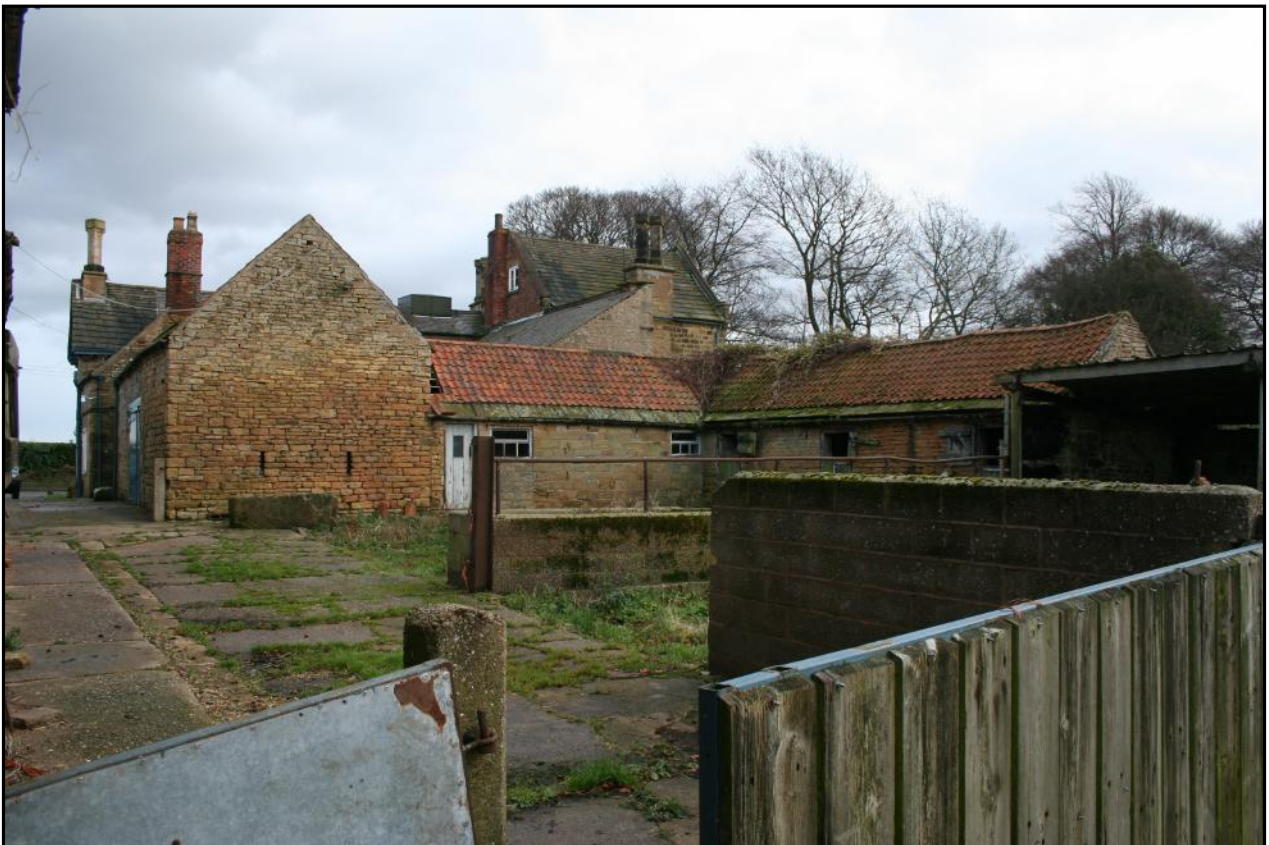
Plate 24: Buildings, now mainly disused, to the west of the large former farmhouse known as The Hall (showing in background) at Hall Farm, Rowthorne.
