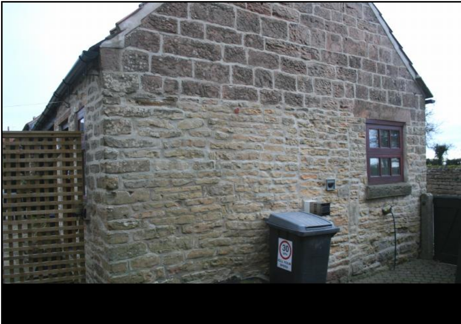
Plate 4: The south end of Structure D at Pear Tree Farm, Rowthorne, showing a blocked doorway in possibly 18th century masonry and a rebuilt gable end.
