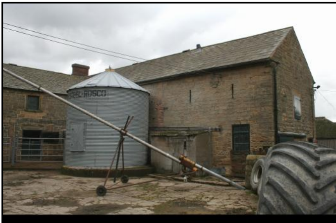
Plate 17: West elevation of the east barn range (C), with a high rounded arch showing behind the tank.
