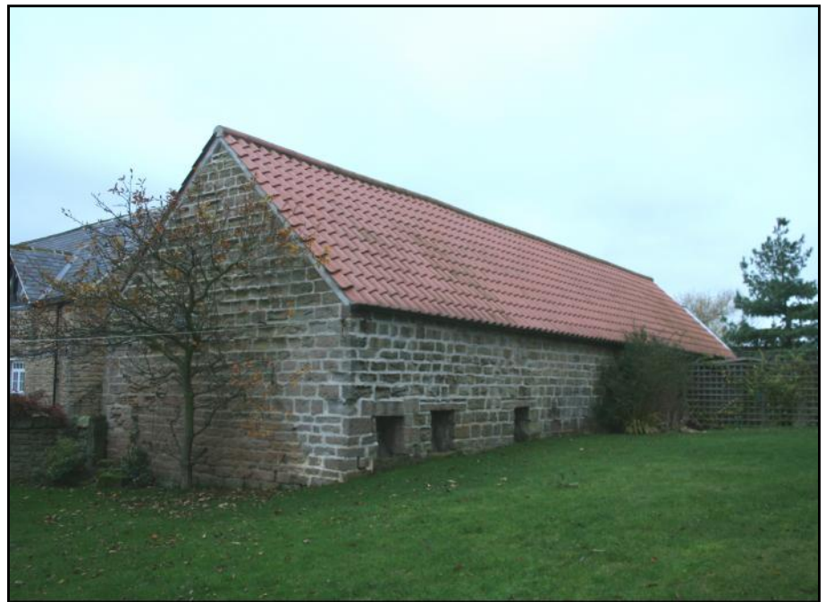
Plate 5: North side of Structure E at Pear Tree Farm, showing pig feeders and a mid-19th century style of masonry,
