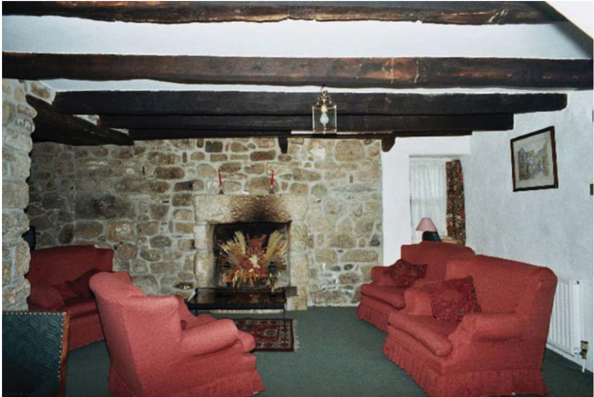
23. Little Keigwin: main front room with later inserted fireplace (note chamfered joists)
