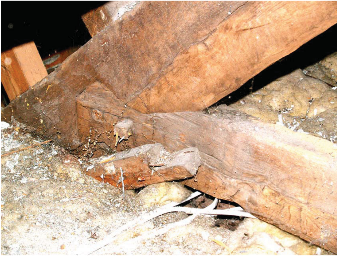
17. Keigwin: front roof structure with detail of collar joint and evidence for former barrel ceiling
