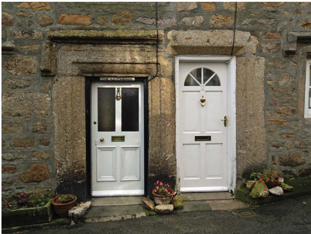
6. The Old Standard: original doorway (left) and later doorway of reused material
