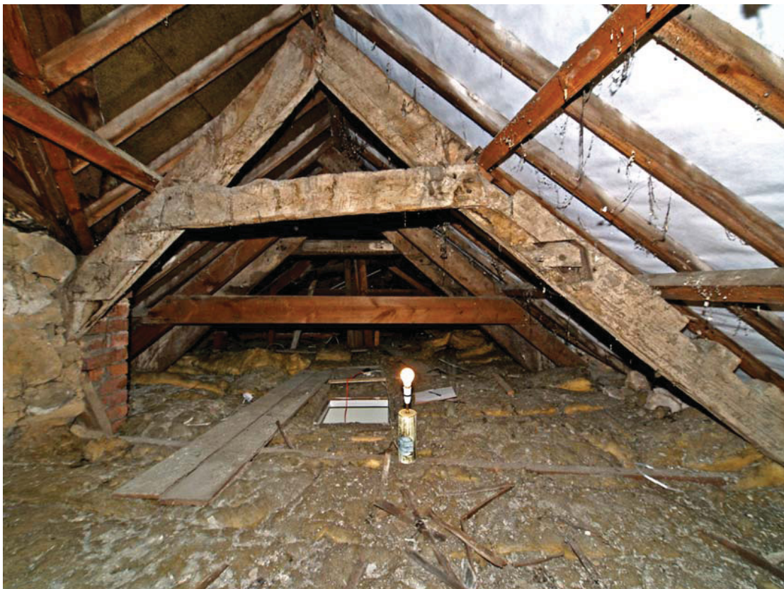
20. Keigwin: roof over east extension to rear range originally with for 2 tiers of collars
