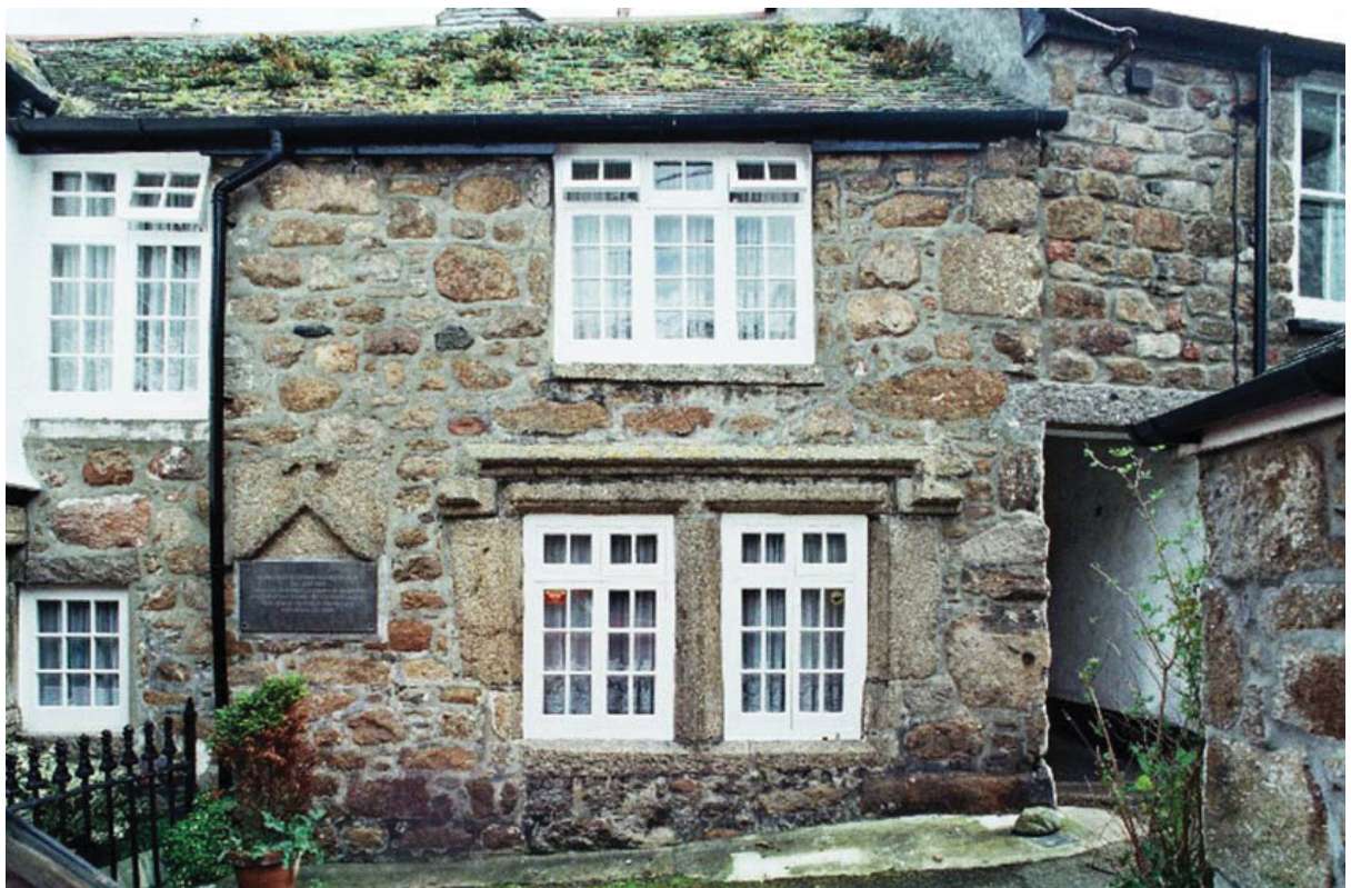
4. Keigwin: restored hall window and reset gable coping of former lateral stack
