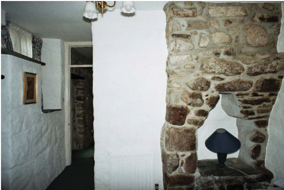
28. Little Keigwin: 18 th century oven inserted to 17 th century fireplace since mostly removed
