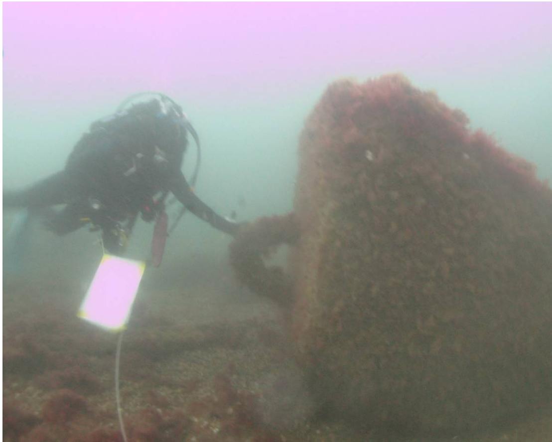
Figure 11. Concrete mooring block.
