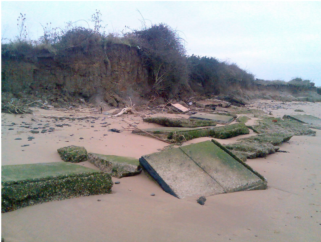
Erosion at Naze cliffs including the remains of a pill box, fallen onto the beach Photo courtesy Bill Wilkinson
