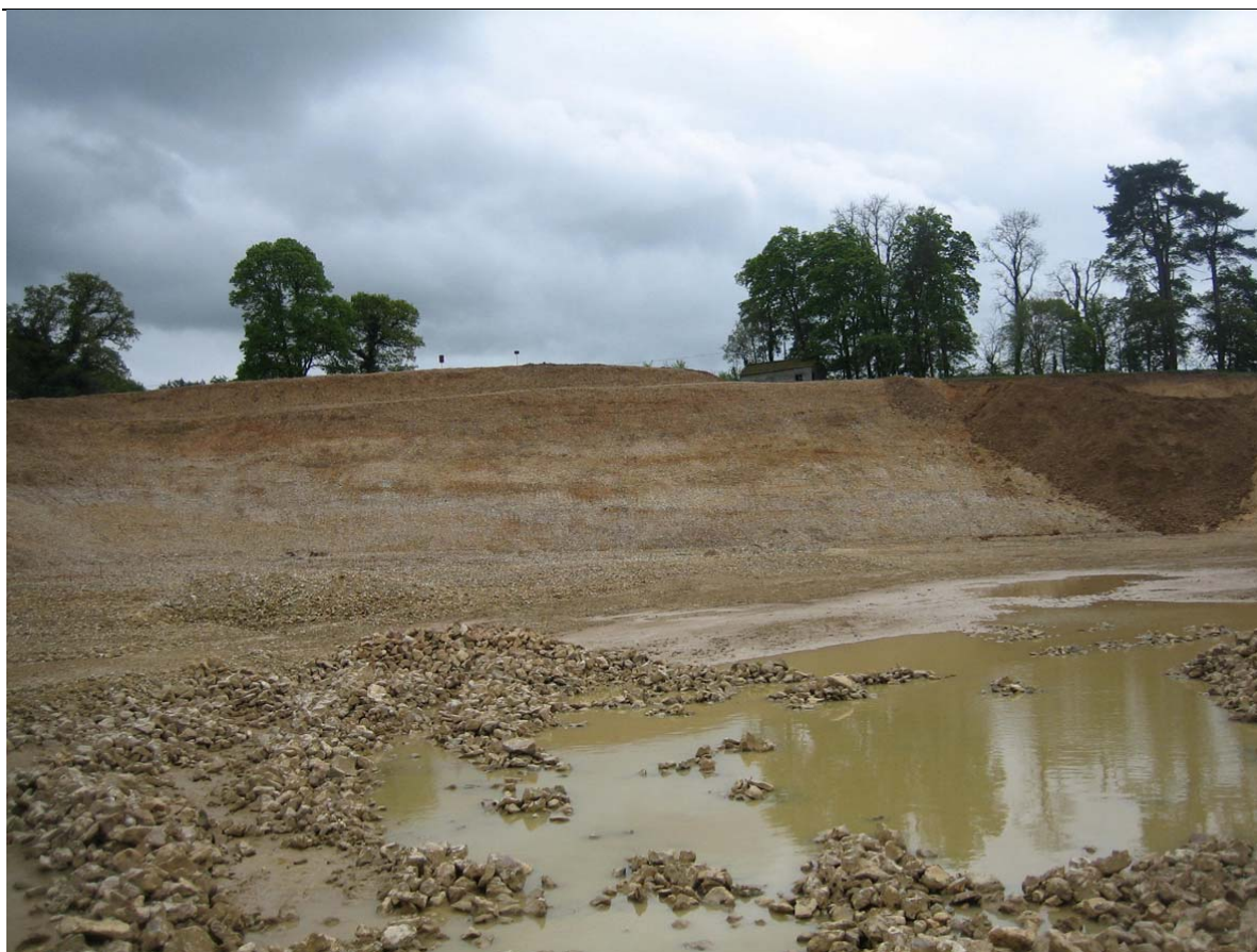
Figure 30 Hodge Ditch Phase 1 at the end of May 2009 looking north. Photo L S Basell
