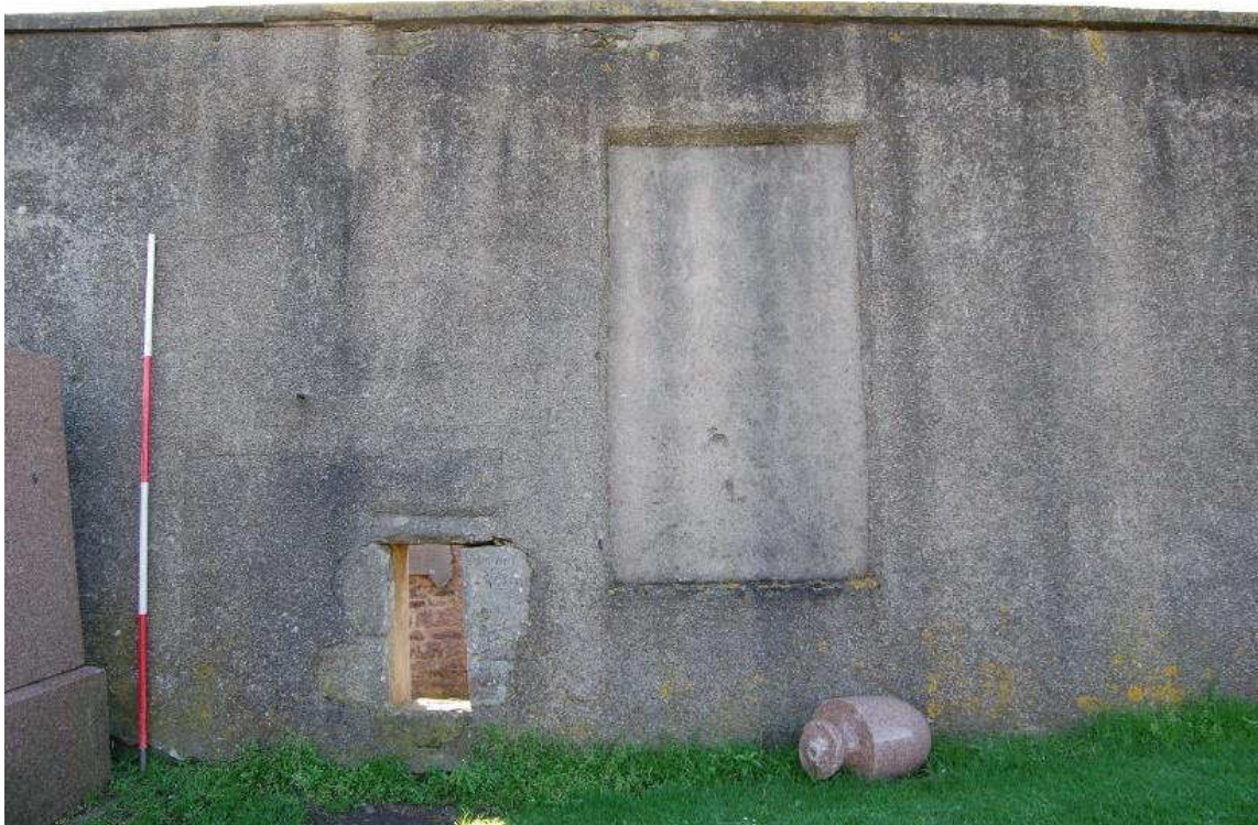
Illus 53 North wall: W4 (just left of centre) with scar of W6, left and infilled window W3, right
