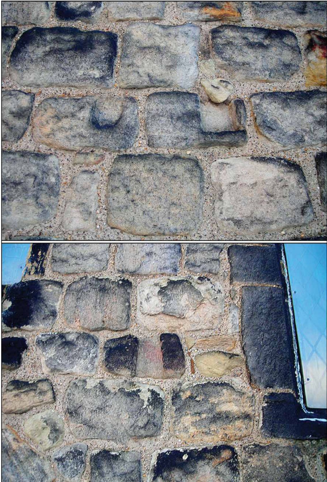
Figure 11: Roman cut mouldings, visible on north external elevation of the Eastern Church at Jarrow.
