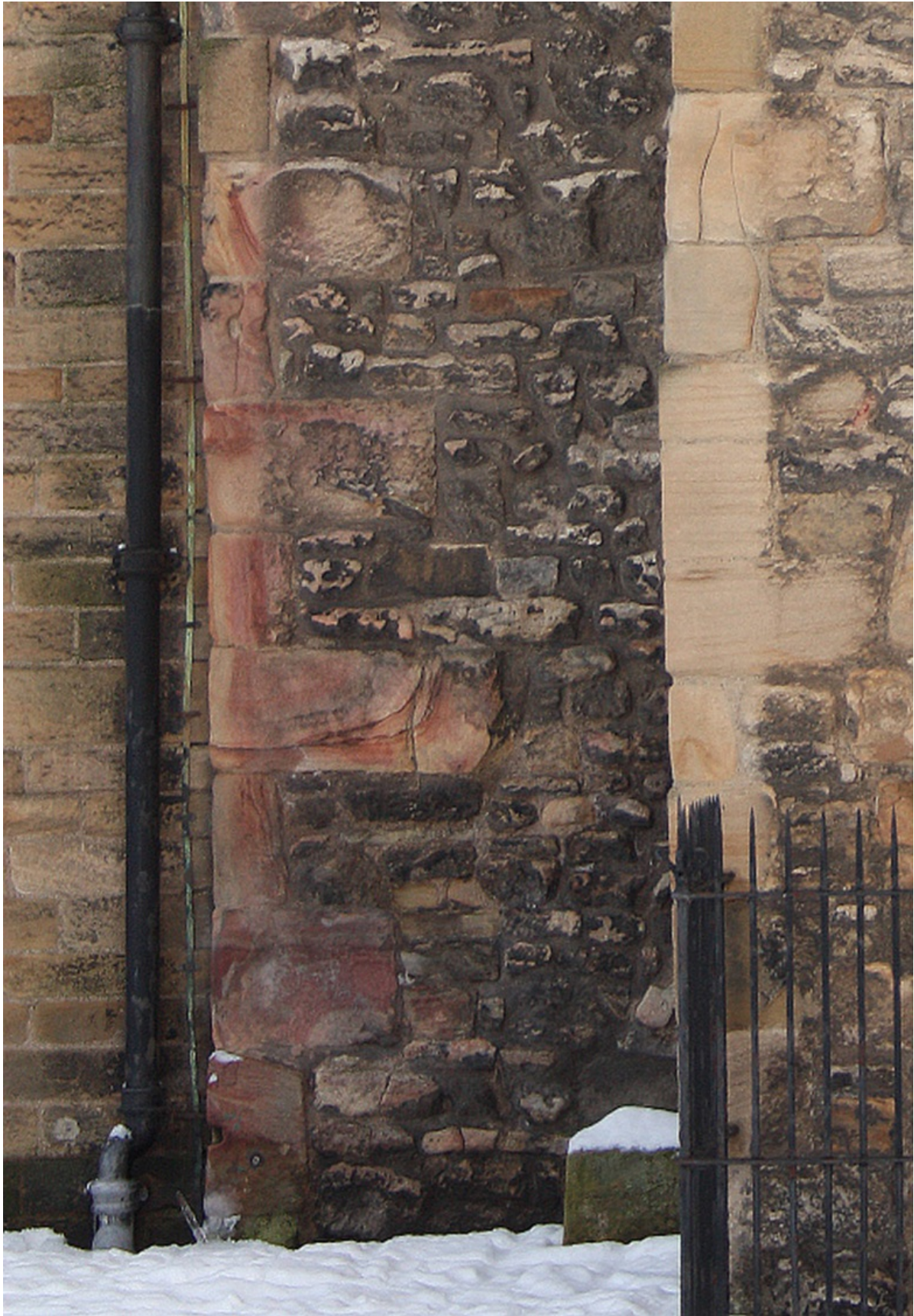
Figure 4: Original quoins at north-west corner of the original nave at St. Peter's, Wearmouth. Note the burned stonework
