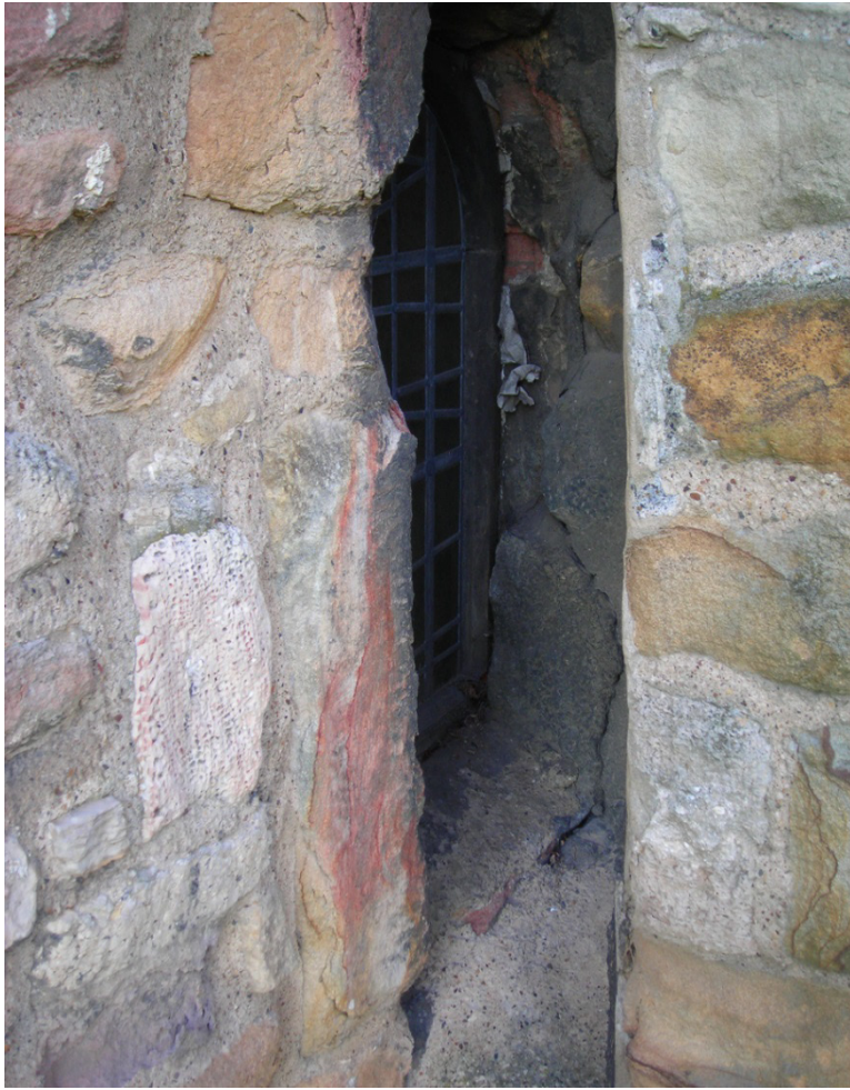
Figure 41b: Fire damage evident on the interior stonework in the western end of the nave at St. Peter's, Wearmouth.
