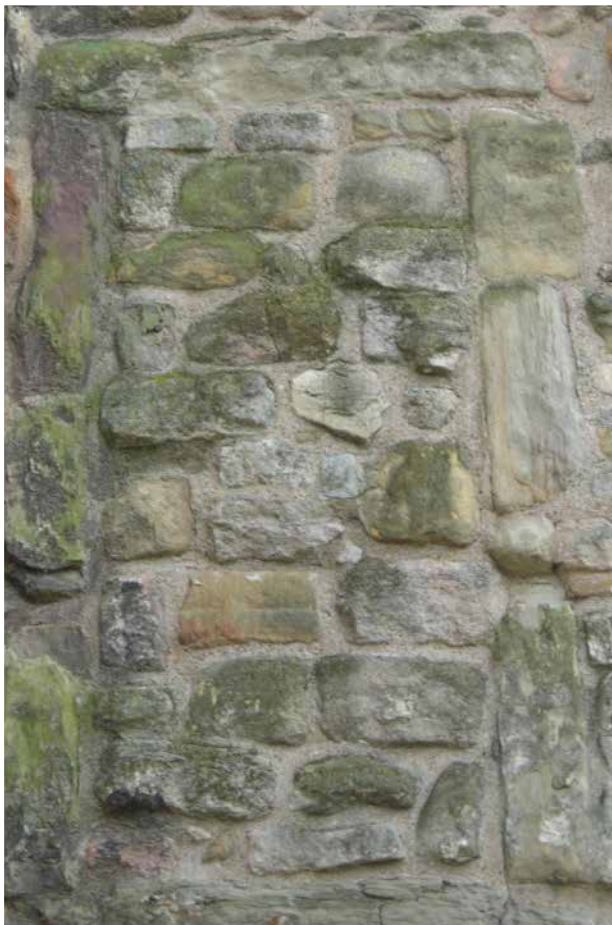
Figure 36: Soft Upper Carboniferous sandstone from the North Hylton area of Sunderland, used in the standing fabric of St. Peter's Church, Wearmouth; above) detail of the poor quality of this ashlar
