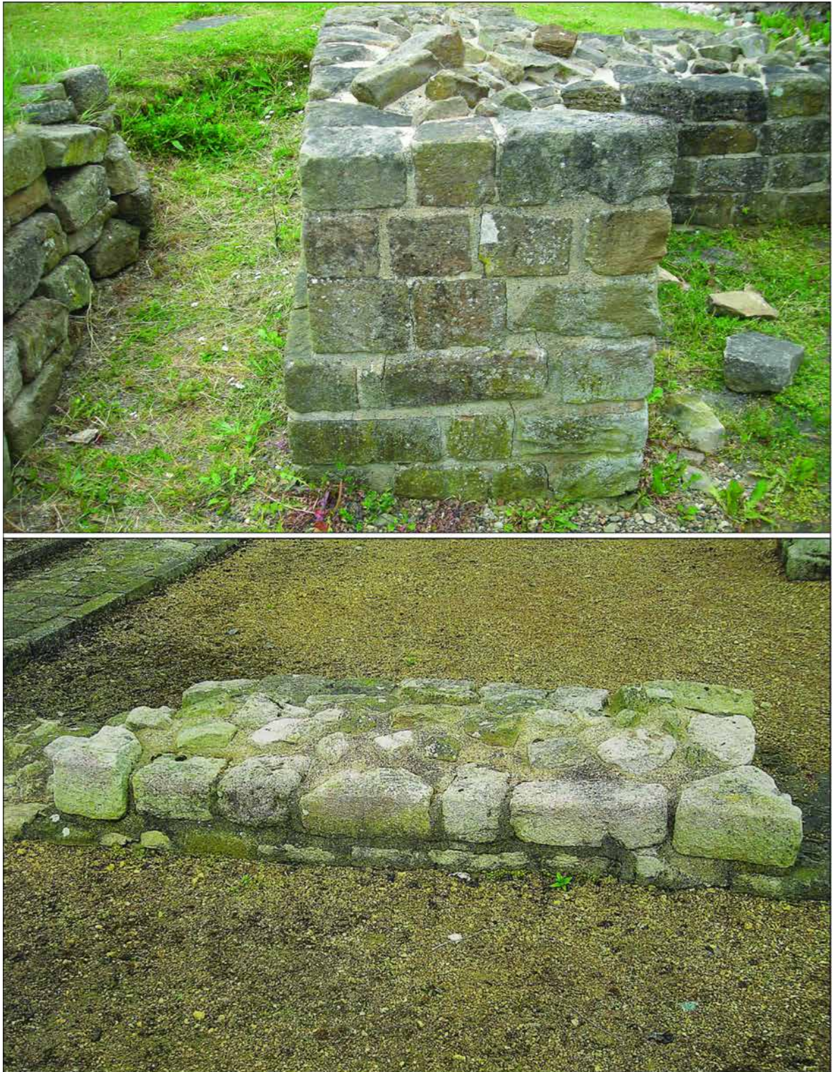
Figure 17: Top: Arbeia: standard 25 x 25 x 25cm squared ashlar executed in Wrekenton Sandstone. Bottom: Segedunum: squared rubble walling executed in Millstone Grit with a lift height of c. 15 cm
