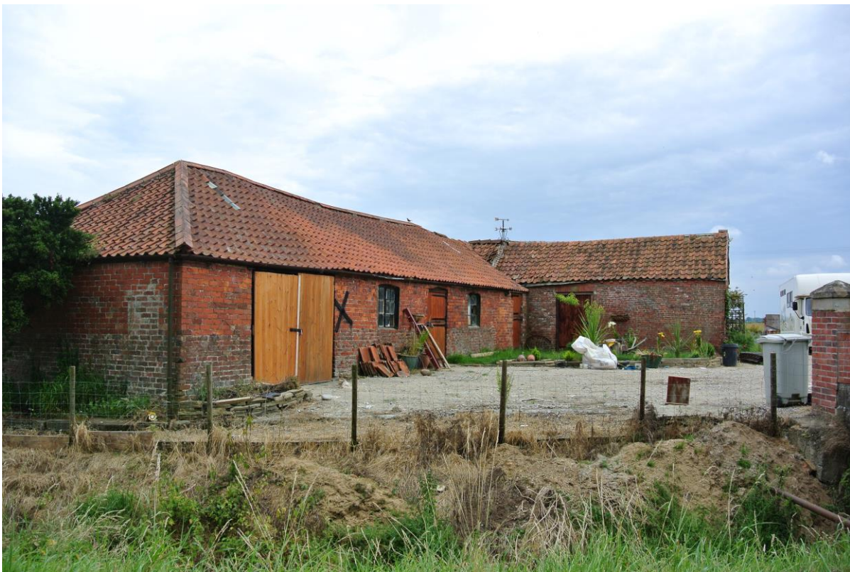
Small L-Plan range with detached farmhouse near Trusthorpe. The materials used here are characteristic of historic farm buildings in the area, although the effects of damp on the brick walls are clear to see
