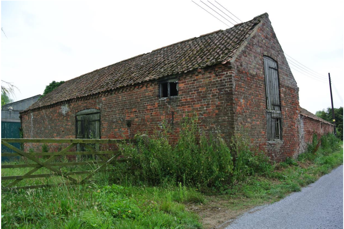
Disused threshing barn, Donington Fen. The barn comprises one side of a regular L-plan courtyard with cattle sheds in the adjacent range, indicating a typical mixed/arable farming operation. The farmhouse itself is set behind the complex facing into the wider landscape and away from the working buildings
