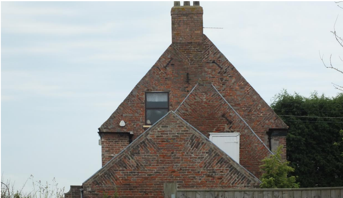
Many gable ends display the traditional tumbled eaves common to the area on 18th and early 19th century domestic and agricultural buildings. (Photo © Jen Deadman)
