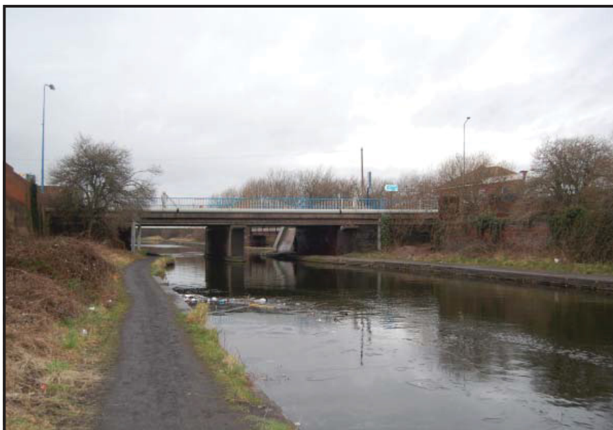
Plate 47: Rubbish in canal.
