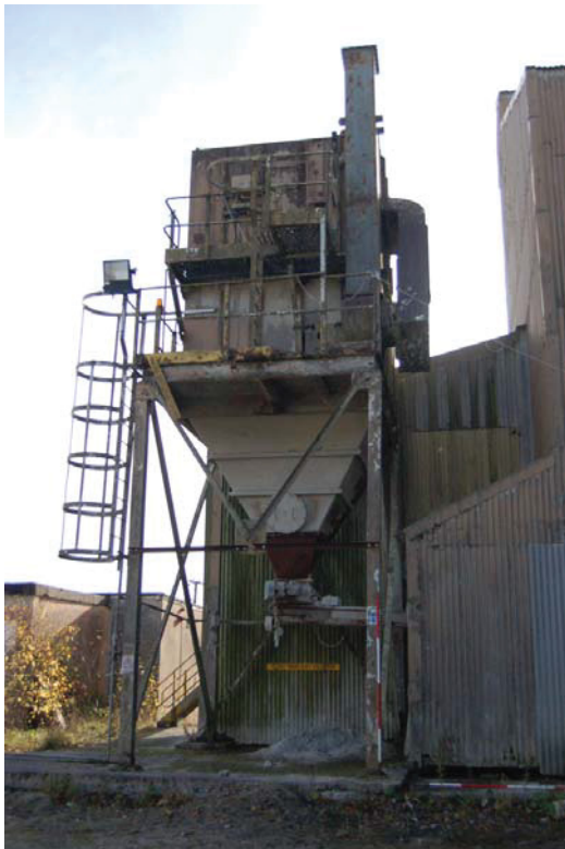
Plate 15: Building [10], 'Nailsea Dust Collector Fan (adjacent to Lanway 4 Crusher). NT SMR 53,209 . View from north-east.
