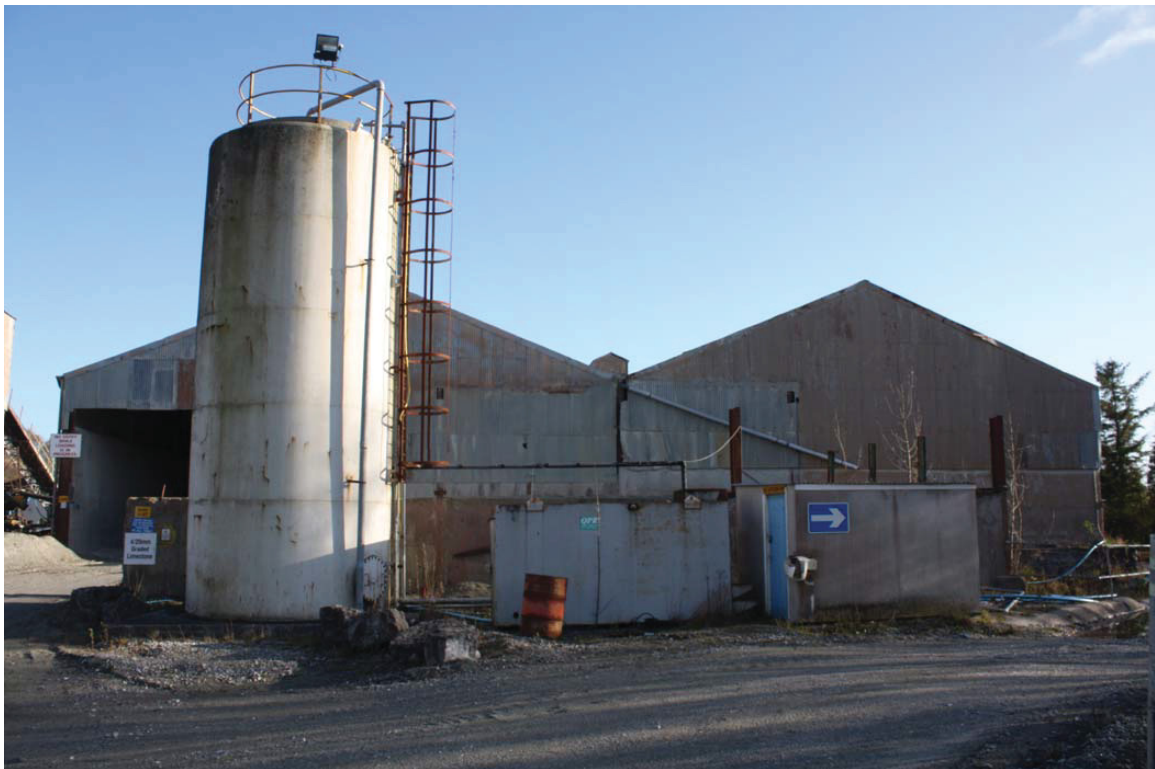
Plate 38: Dust Suppression Pump and Tank [29], NT SMR 54,228 . View from south-west.
