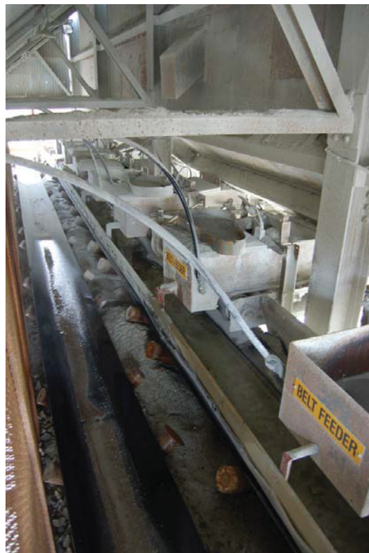
Plate 20: Grading Plant [13], interior Detail of belt feeders.
