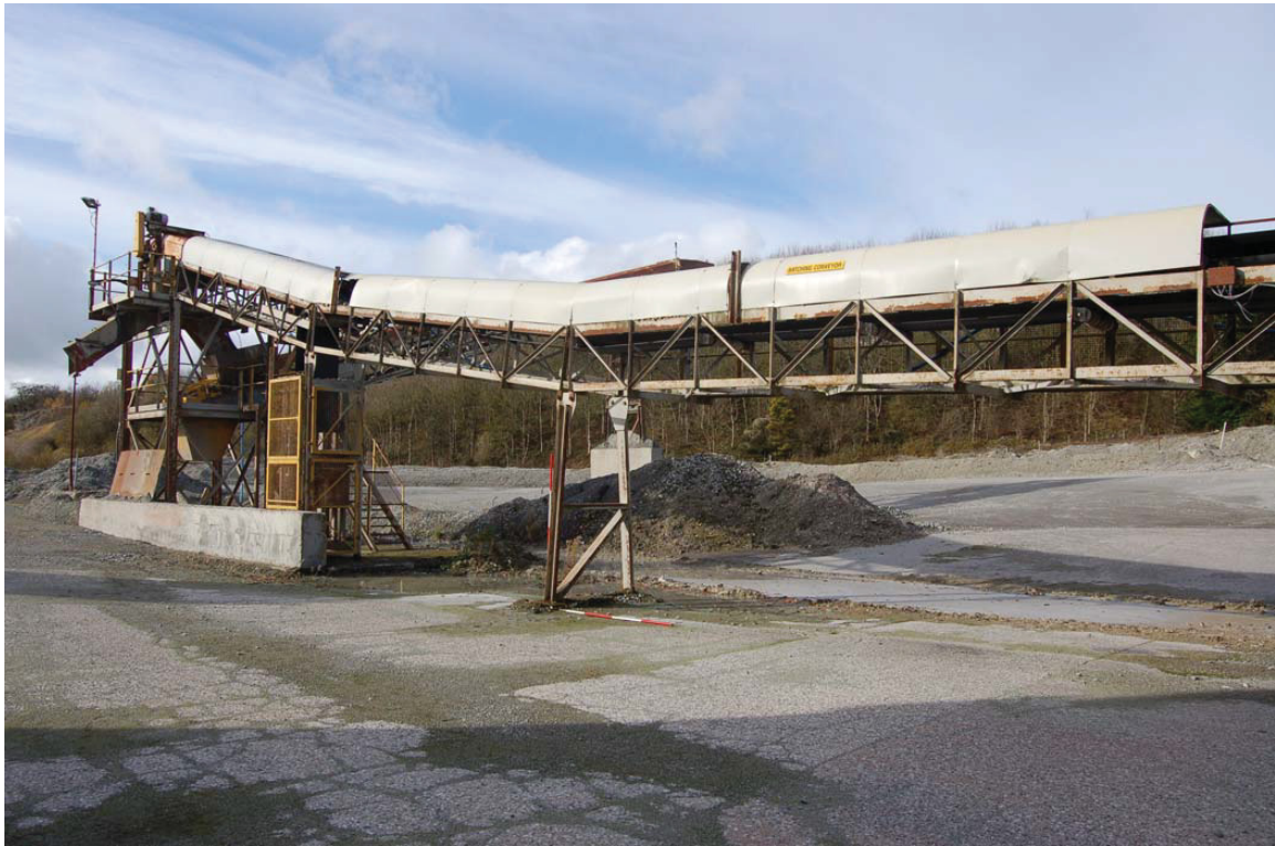
Plate 23: 'Batching Conveyor' [16] (NT SMR 54,215) and Loading Chute [17] (NT SMR 54,216) (left). View from east. (see also Plate 15).
