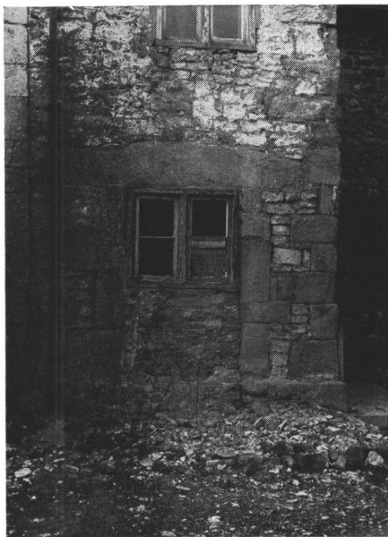
b. Exposure of the porch door.
