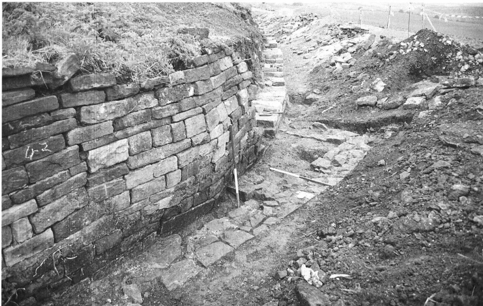
Plate 5: Sutton Scarsdale Hall: drystone-walling of the ha-ha (intact at left, under repair at right), with the levelled footings of earlier mortared walls in the foreground; looking north-west; scales 1m. Photograph by R. Sheppard.
