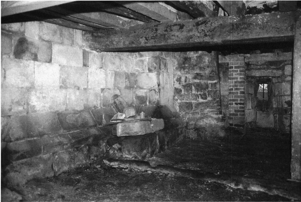
Plate 1: Breadsall Old Hall: a corner of the undercroft, showing (left to right) the plinth of an earlier building, the enclosing wall of a spiral stairway, and a Medieval splayed window contemporary with its wall; looking south-east. Photograph by R. Sheppard.
