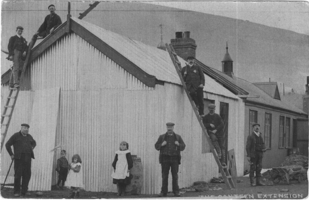
Plate 5: The Derwent Canteen during construction work to extend it. © Prof Brian Robinson.
