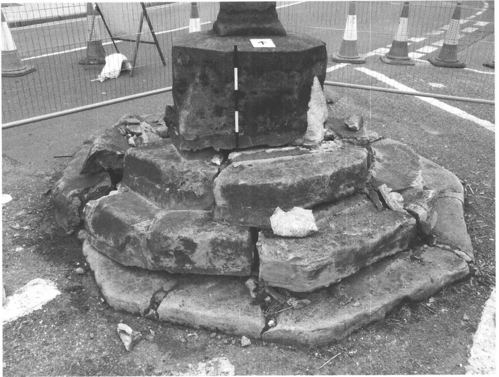
Plate 5: Clowne Cross: the cross showing, to left, the displacement of its stepping stones after vehicle impact.
