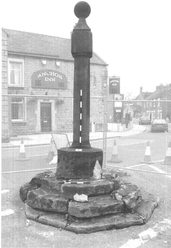
Plate 4: Clowne Cross: the damaged south side of the cross's steps after vehicle impact.
