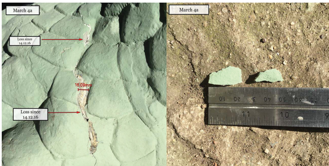
Plates 27 and 28. Crack 4A – Photographed 15.03.17 – disassociated losses incurred since 2016.
