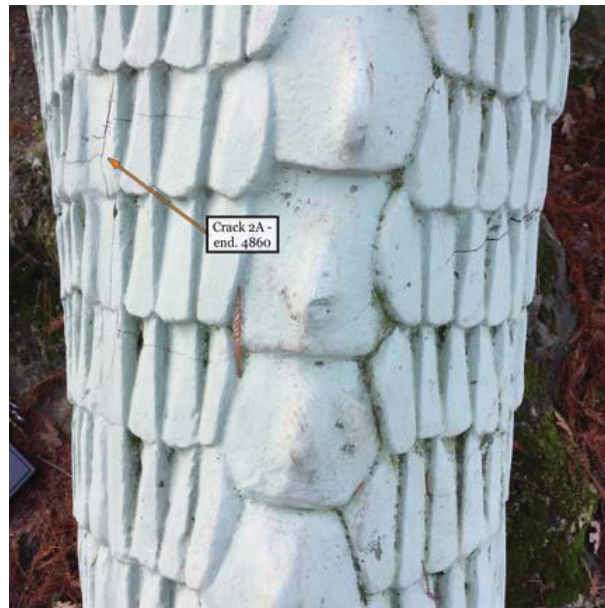
Plate 16. Photographed 14.12.16 – End measurement point of Crack
