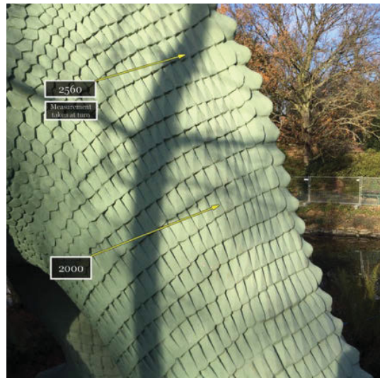
Plate 7. Photographed 14.12.16 – Crack 1A
