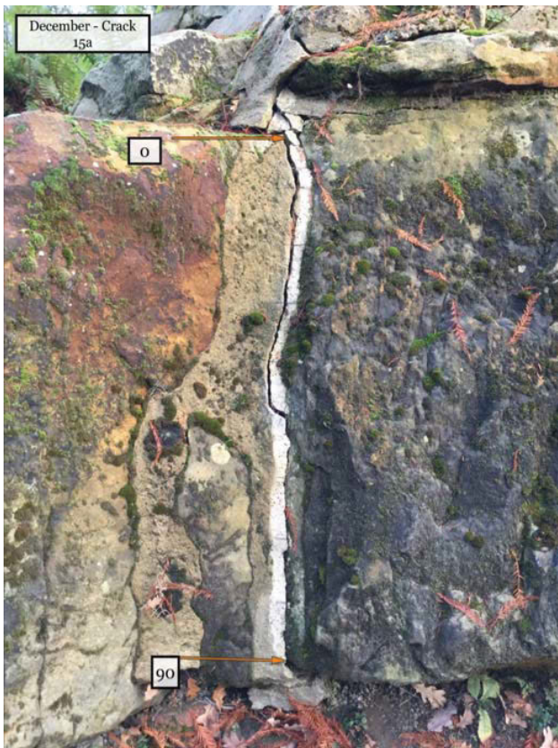
Plate 43. Photographed 15.12.16 – Crack 15A.
