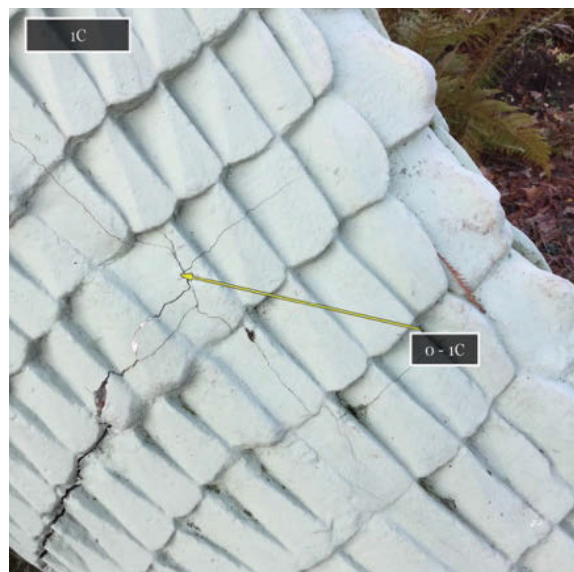
Plate 9. Photographed 14.12.16 – Crack 1C.
