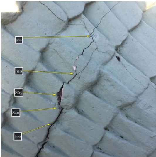
Plate 6. – Photographed 14.12.16 – Crack 1A.
