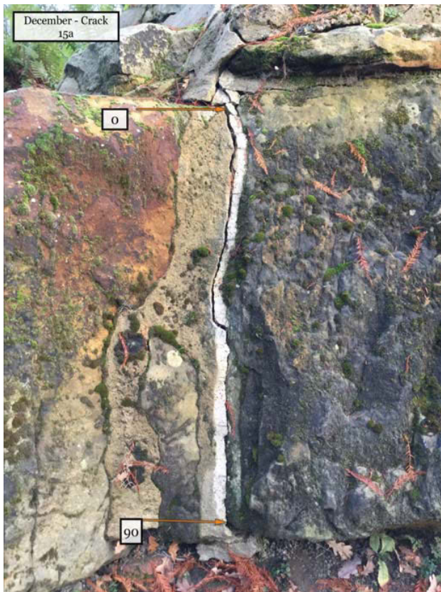
Plate 105 - Photographed 15.12.16 – Crack 15A 80
