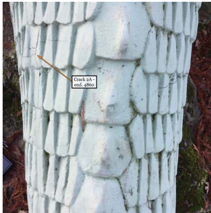
Plate 64-. Photographed 14.12.16 – End measurement point of Crack 59
