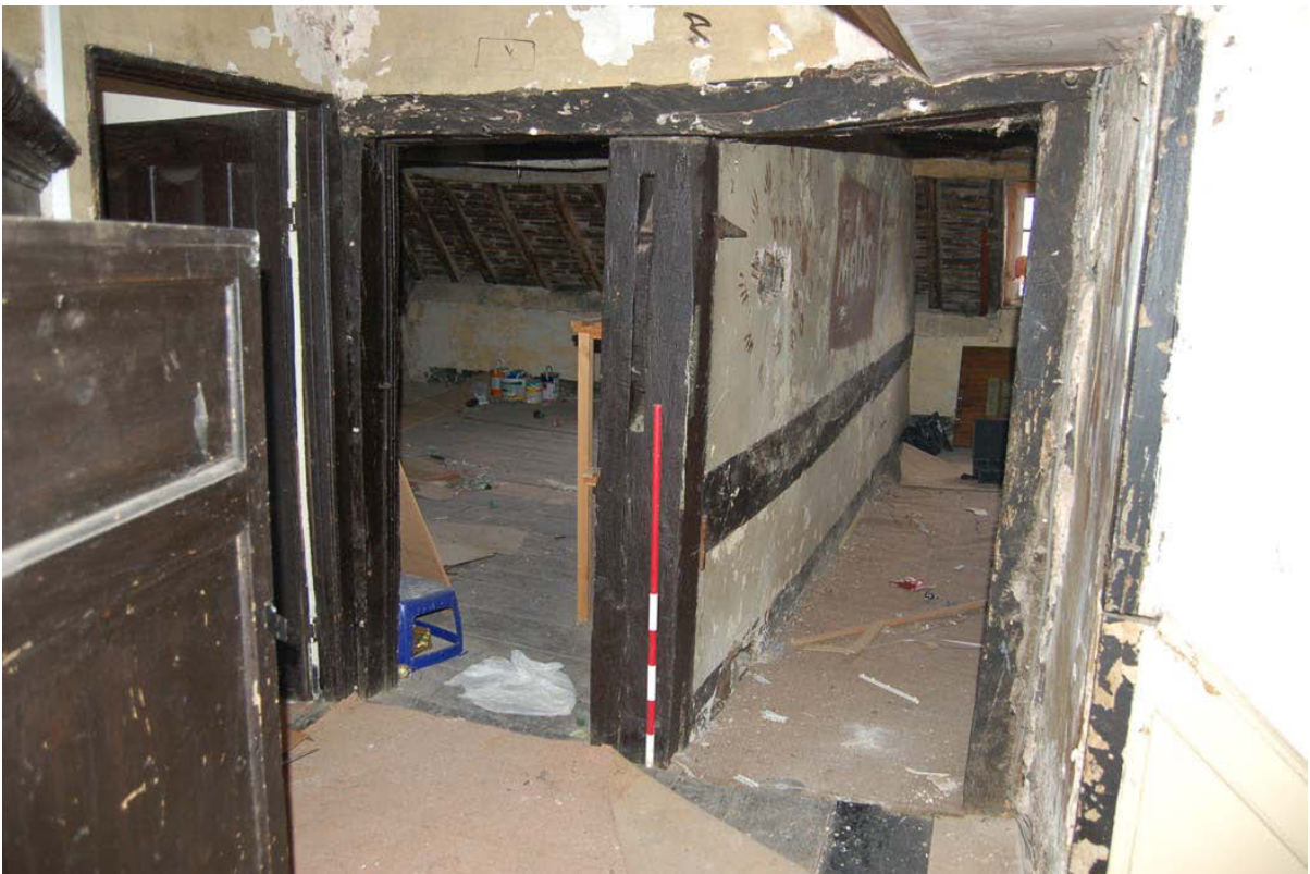
Plate 62: Doors to T4 (left) and T1 (right) at head of Stair B.
