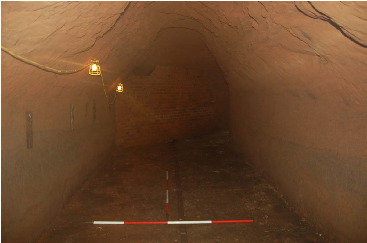
Plate 21: Chamber S1 looking south, note brackets on east wall (l.) and angled brick partition.
