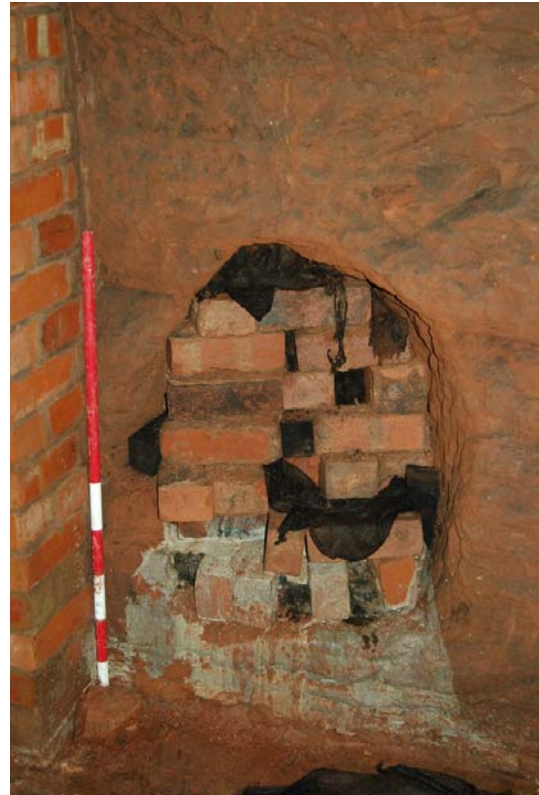
Plate 57: N2, blocked communication tunnel.
