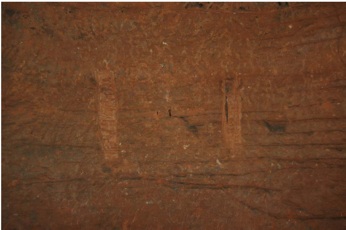
Plate 41: Chamber S4 south end; vertical scars in end wall.
